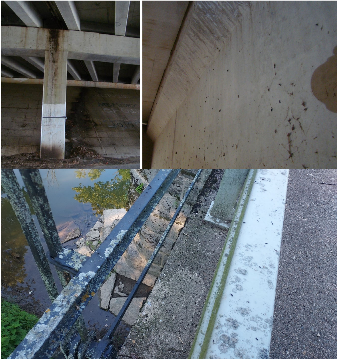
Figure 12. Examples of guano accumulations on bridges. (photos provided by Georgia Department of Natural Resources (top) and Indiana Department of Transportation (bottom)).
