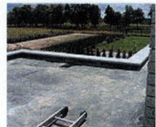
An EPDM rubber roof
