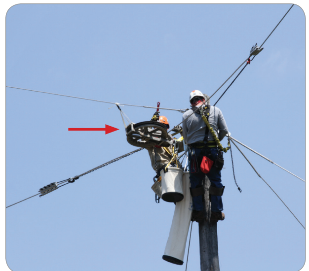
Figure 4—Tying a support rope to the sheave keeps it suspended to the stringing block.
