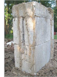
Mud tubes on a block pier
