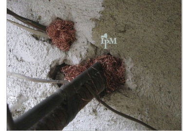
Gaps stuffed with copper mesh
