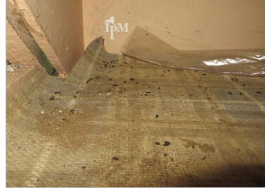
Mouse droppings along a wall
