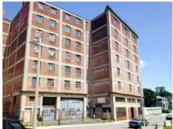
Dilapidated buildings in Roxbury.
