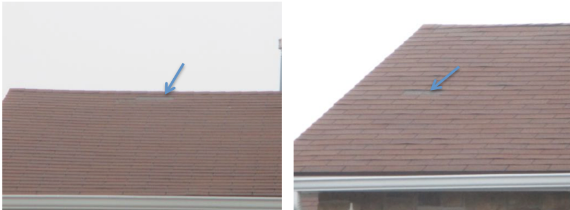
Few missing roof shingles
