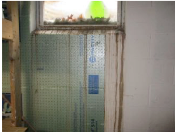
Evidence of leakage at rear basement window
