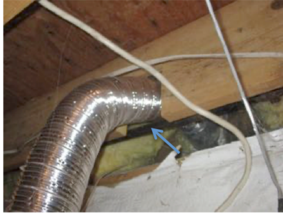
Cut in floor joint above the laundry area in the basement
