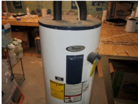
Electric hot water heater
