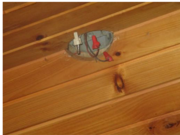
Open junction box above the pool house
