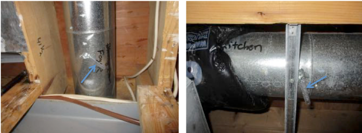
Examples of closed dampers in the basement
