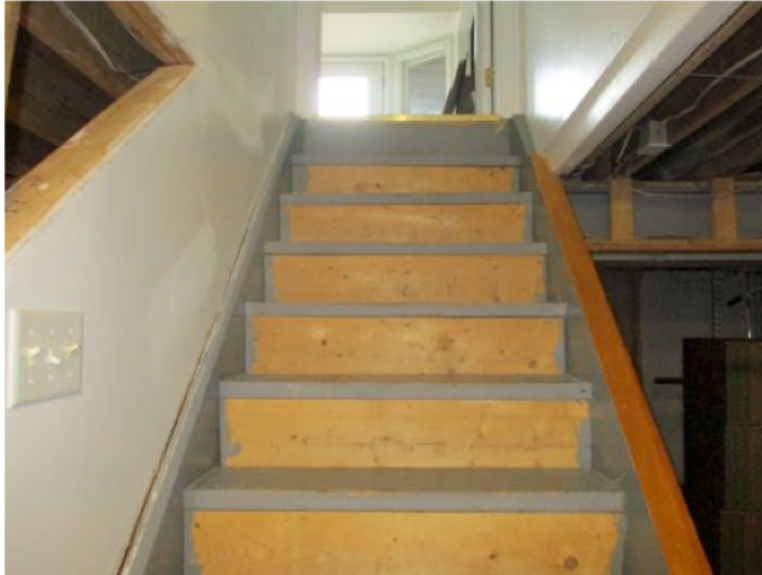
Basement stairs lacks a handrail and a guardrail
