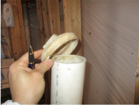
Uncapped waste pipe in the basement
