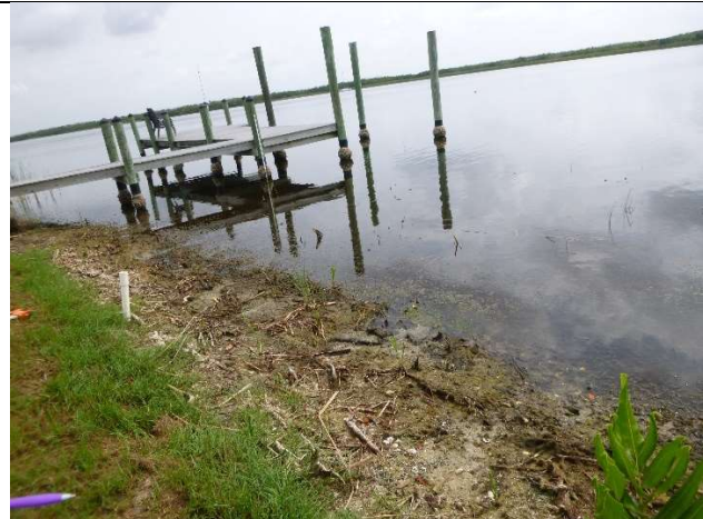
Photo 3: View of unauthorized mangrove removal on Property 1. Facing northeast
