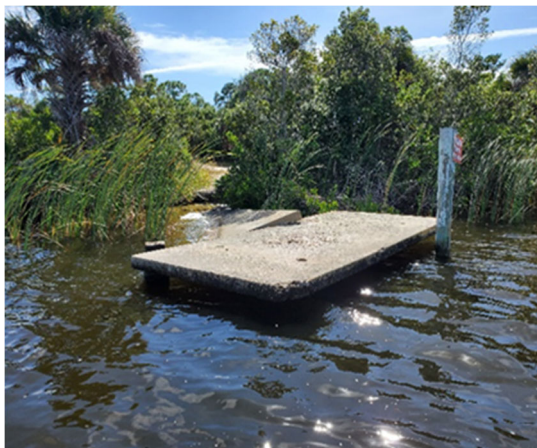
County Code Compliance Violation
