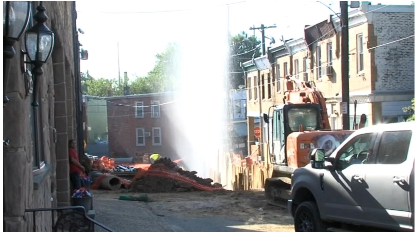
Construction crew strikes water main, creates Frankford geyser: as seen on Action News Mornings
