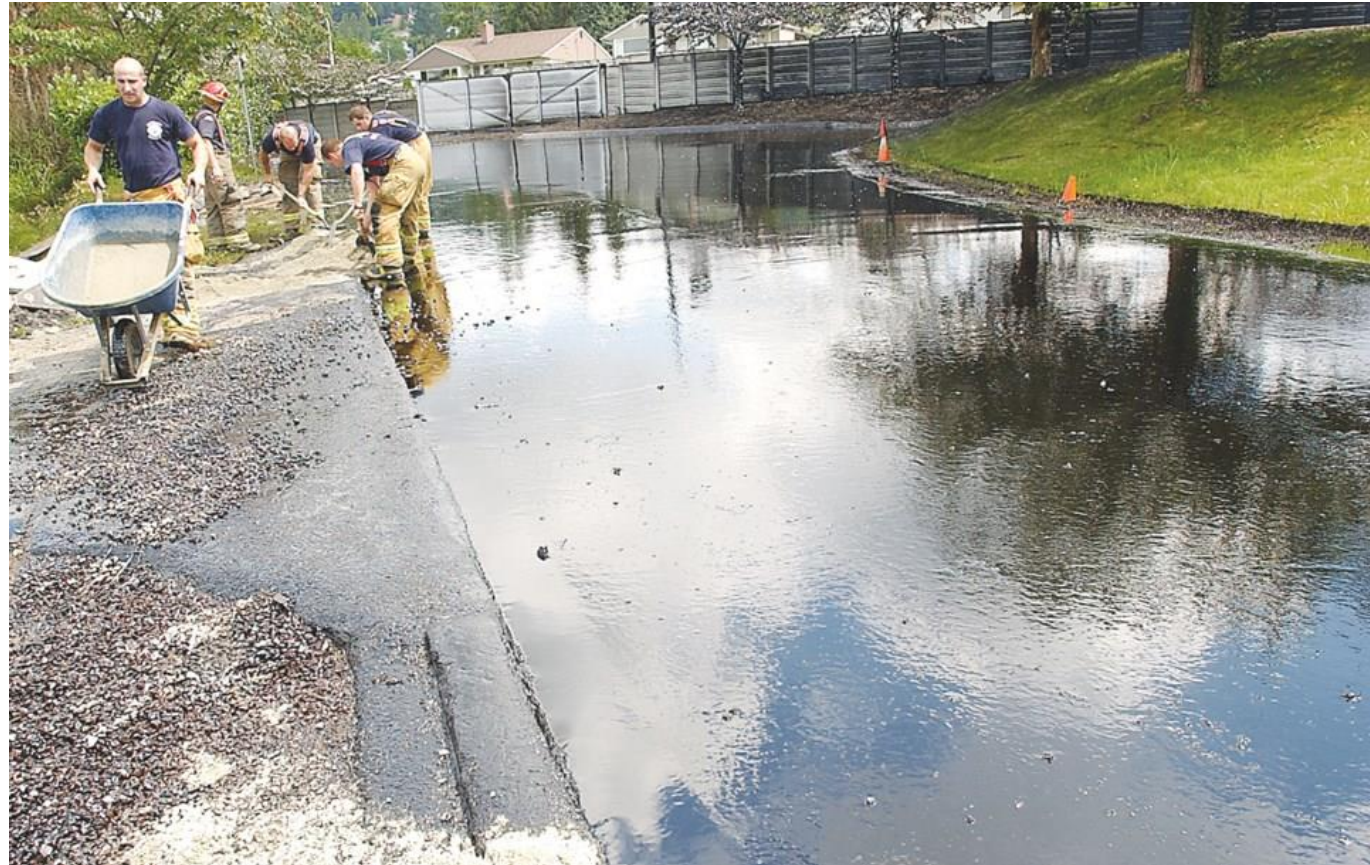
Blocking storm drains on oil spill site to prevent runoff into Burrard Inlet – July 2007 photo by Burnaby Now
