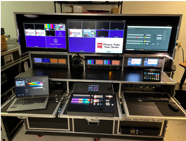
Front View of FLYPACK1 showing the Blackmagic Control Surface, Laptop Drawer, Streamdeck, and monitors.
