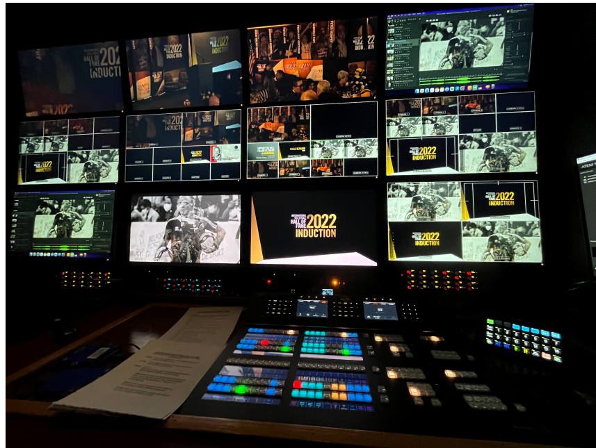
TD Position with Switcher Control Surface and Monitor Wall
