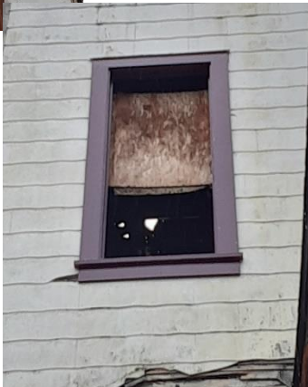
New Window Frame is waiting for new sash. Note daylight where siding is damaged on opposite side
