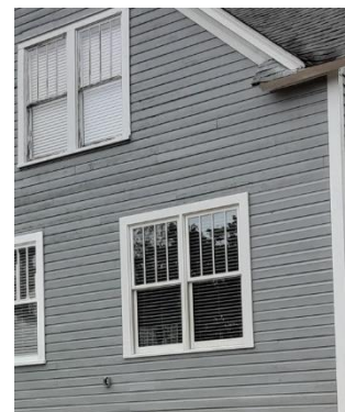
Note the removal of asbestos to expose original wood siding. While portions are new wood, the appearance is traditional.
