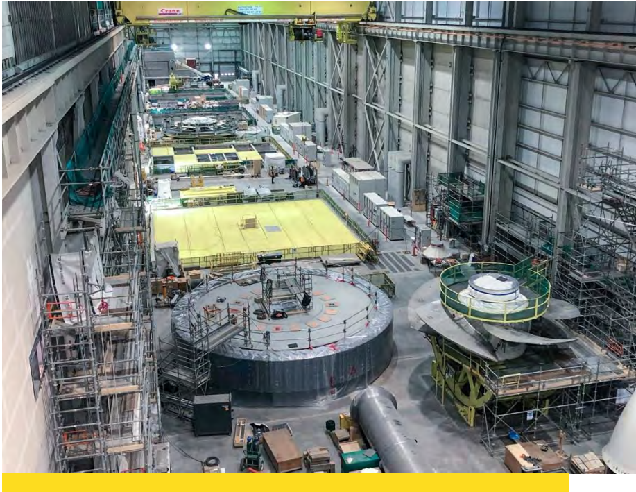
Carillon Power Generating Station, QC, Canada
