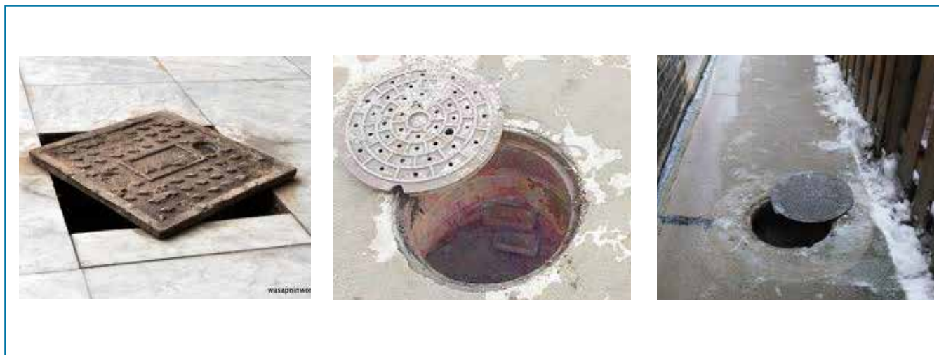
Figure 28: Manhole / Manhole covers
