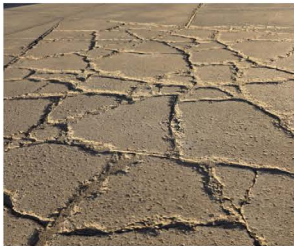
Cracked and broken concrete
