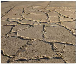
Cracked and broken concrete
