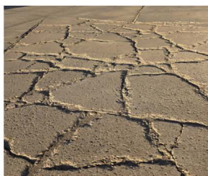
Cracked and broken concrete
