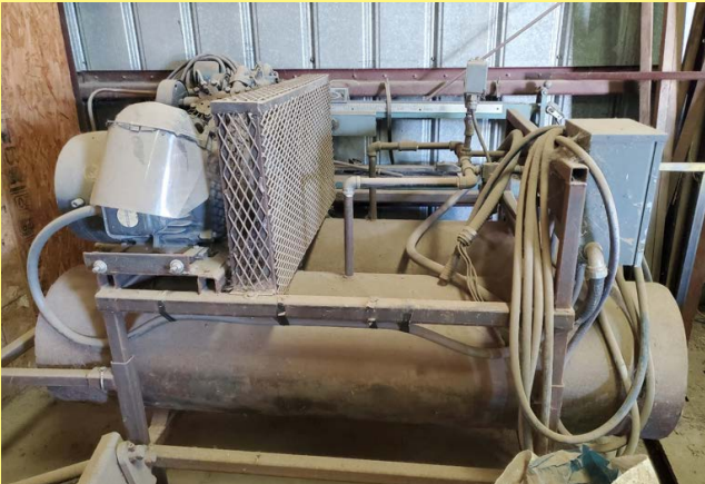
Home Made Air Compressor
