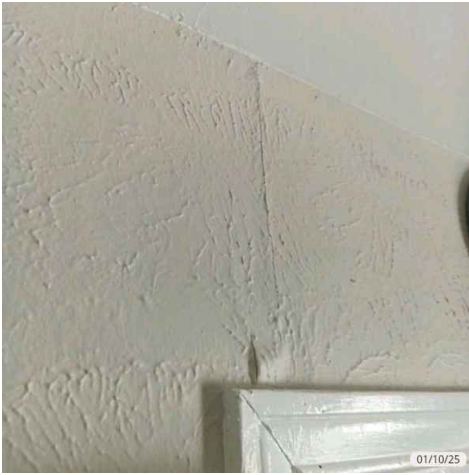
Dining room. Previous patching
