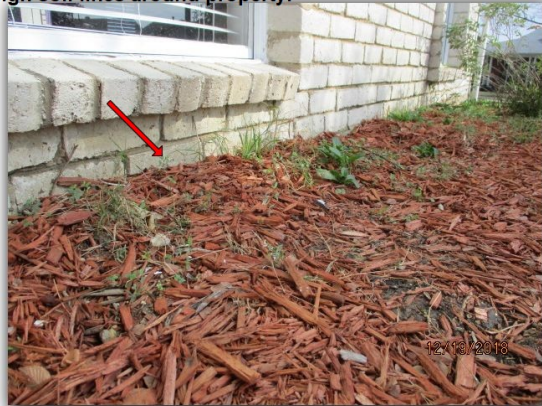
High soil lines around property.
