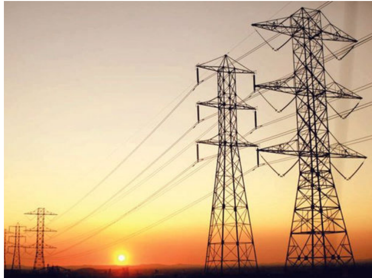
POWER AND TELECOMMUNICATION LATTICE TOWERS
