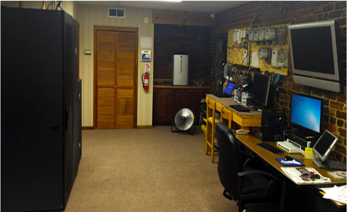
GRID MICRO LIMITED'S SMART AMI ELECTRIC METER LAB
