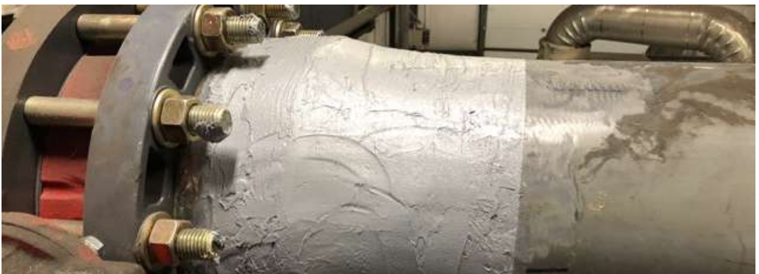
Cooling water line leak stemmed at a power plant
