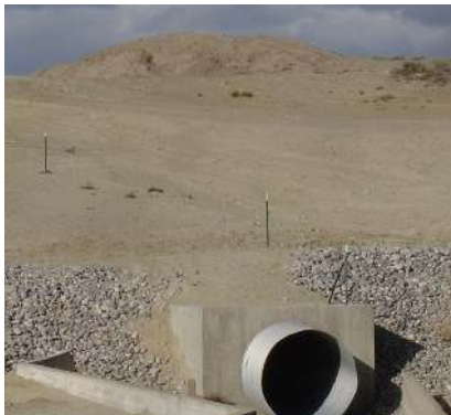
Pipe used to carry irrigation water
