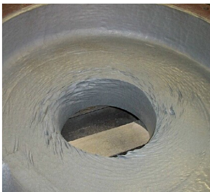
Entrainment damage on slurry pump
