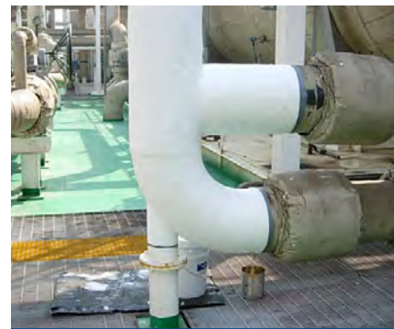
Pipe lagging sealed
