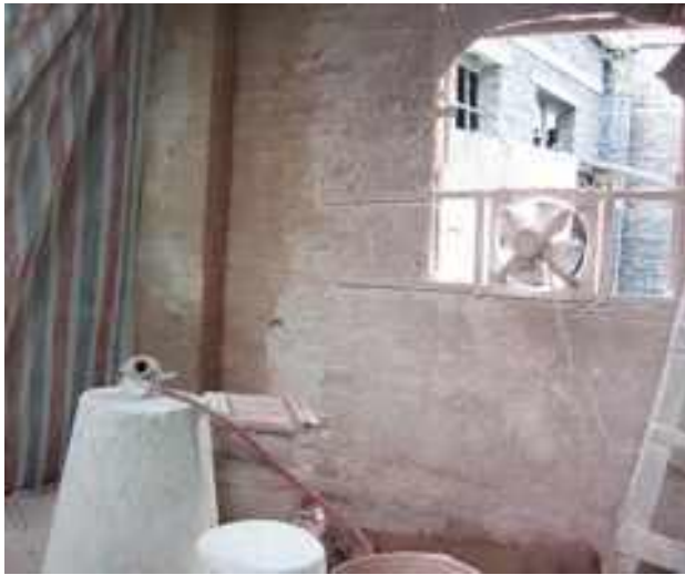
They were all sprayed with glaze. This exhaust fan was a joke.
