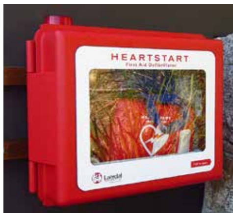
Our defibrillator is mounted on the block wall between 13 and 17 Knowlman Road.
