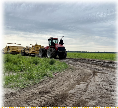
Above: Contractors moving dirt according to NRCS designs to direct water flow into a perimeter ditch
