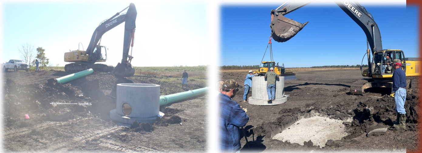
Setting a manhole water control structure on the ~300 acre pool for our Pike County easement
