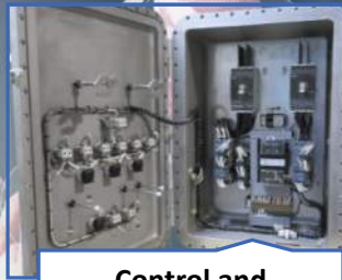
Control and Automation Systems
