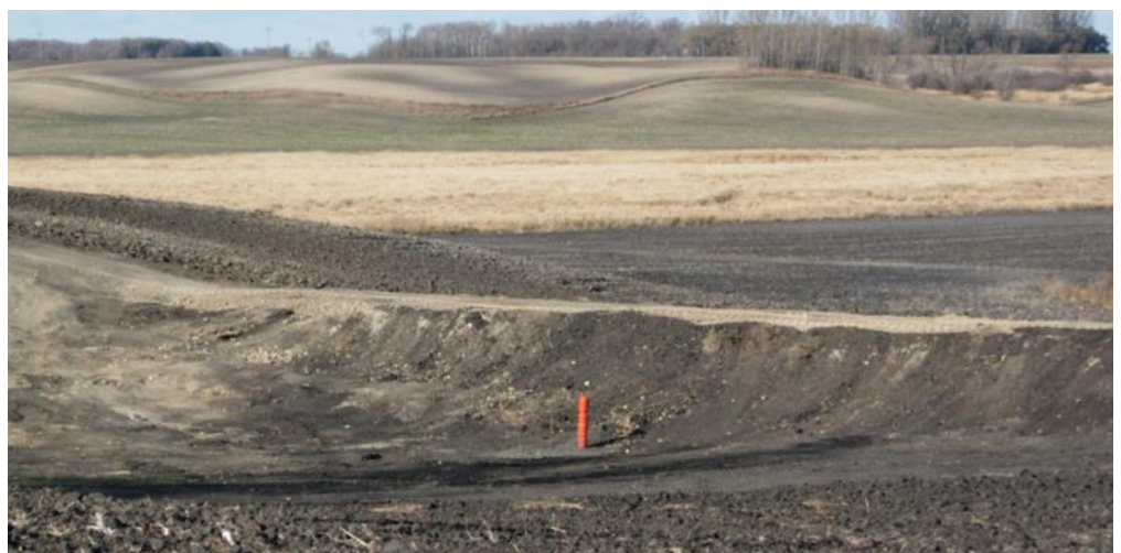
Figure 2: Installed WASCOB with Hicken bottom. Photo credit: East Polk SWCD.
