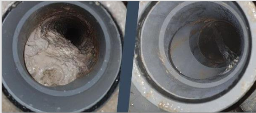
Clean grease buildup and blockages in kitchen oil pipes.
