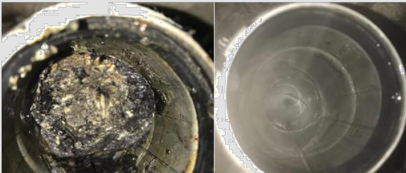
Remove urine scale buildup inside toilet waste pipes.
