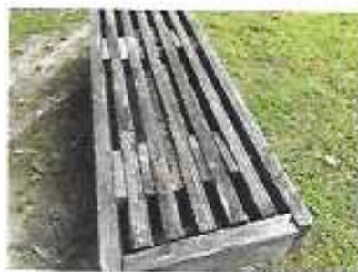
Figure 9 Deterioration Detail, NE Bench
