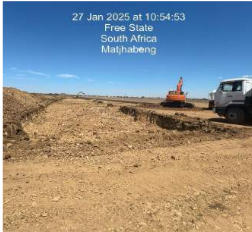
Figure 5: Open trenches must be barricaded.
