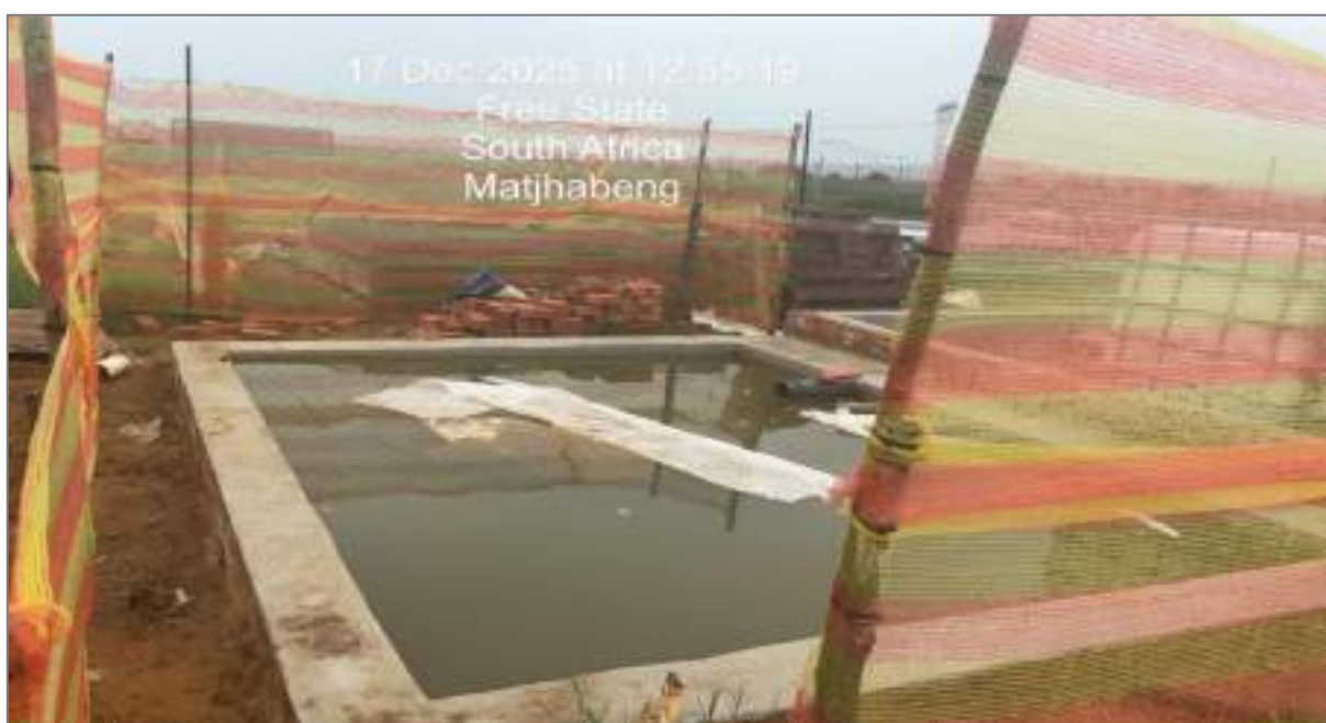
Figure 4: Overflowing sump at the waste area.
