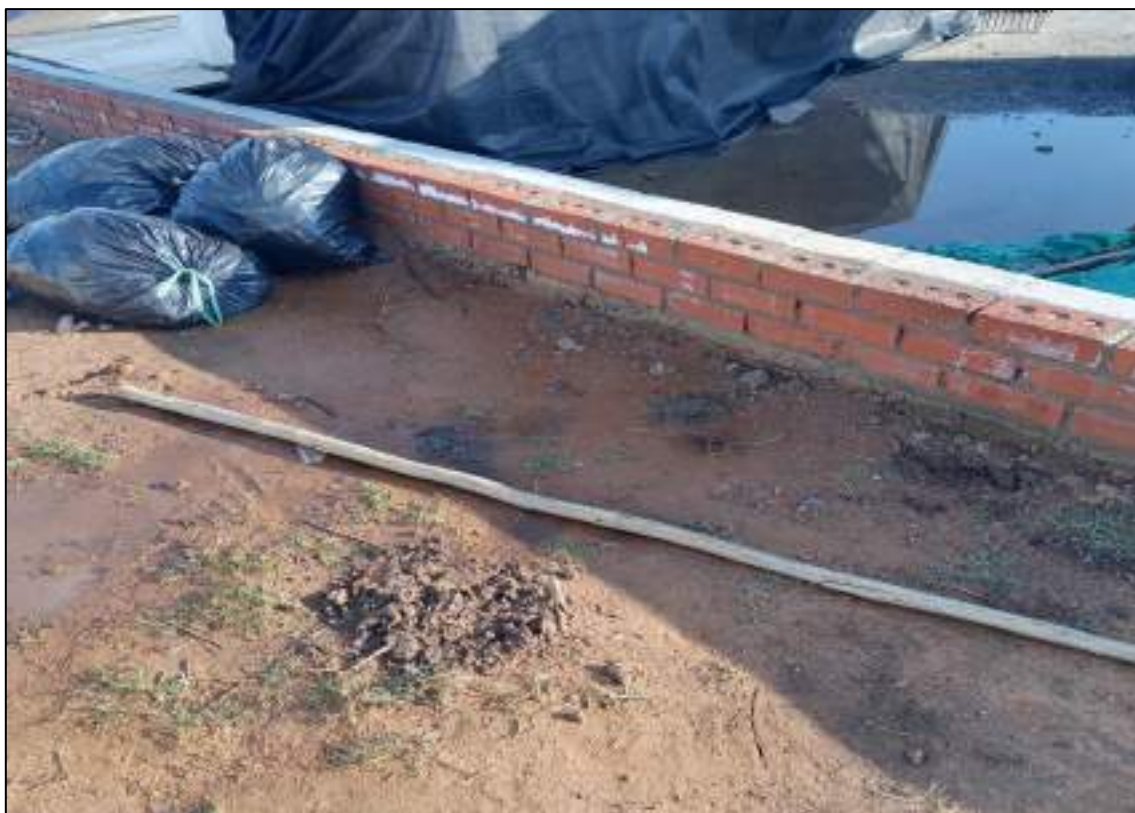
Figure 10: Leaking waste bund
