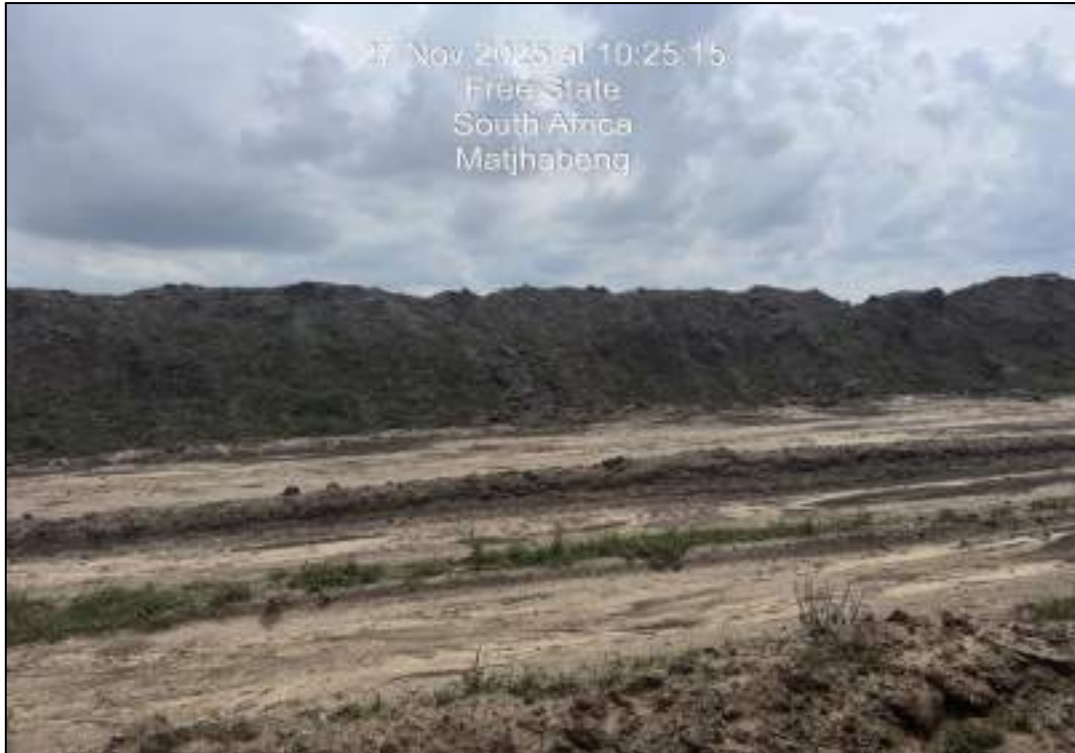
Figure 9: Open trenches left open unbarricaded.
