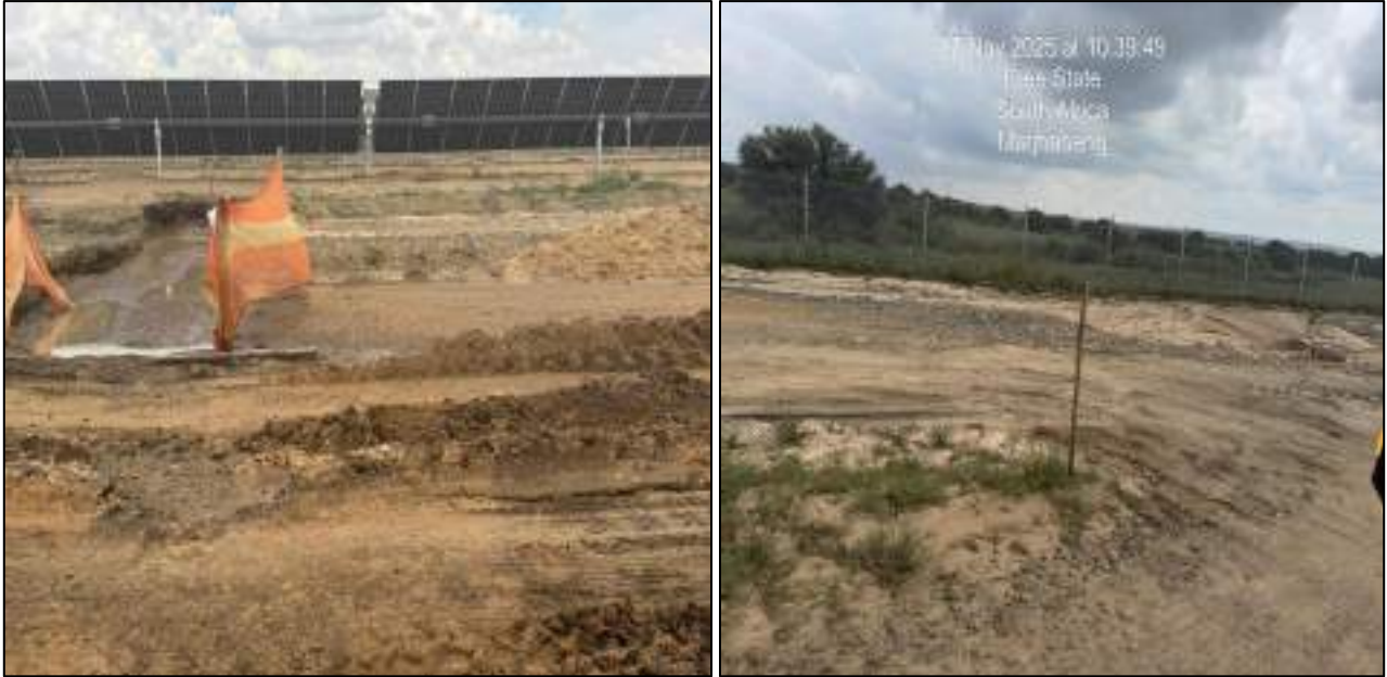
Figure 7: Damage caused rainwater
