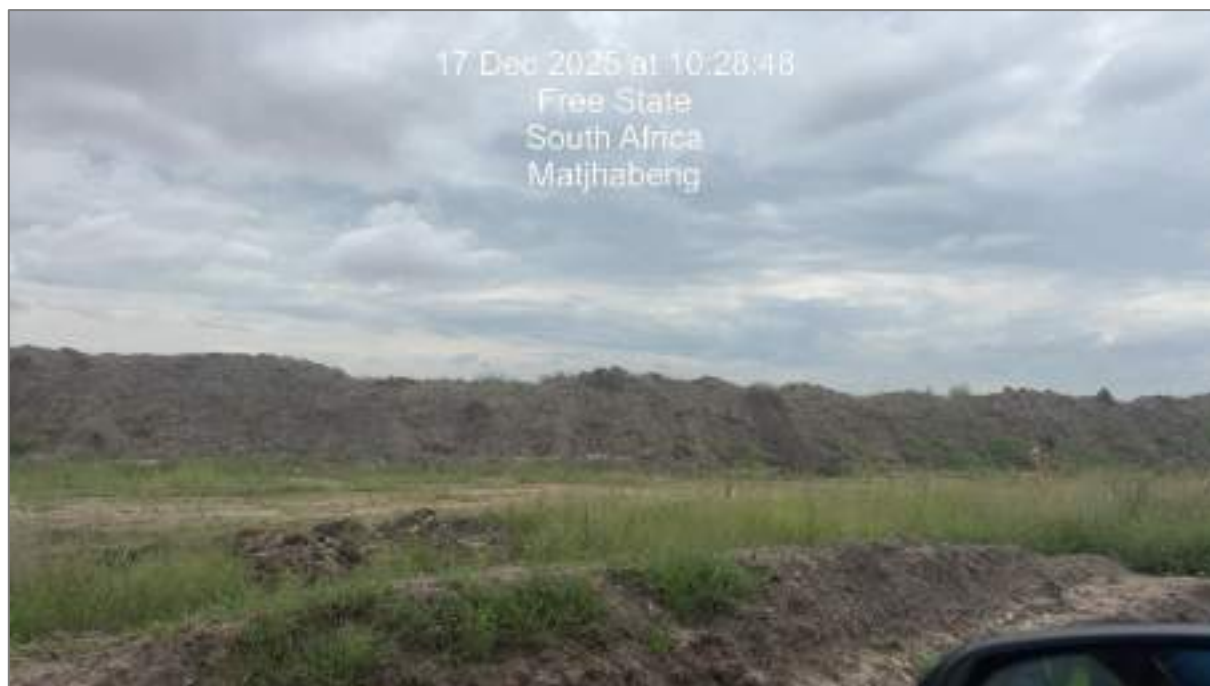
Figure 9: Stockpile height exceeding 2m.
