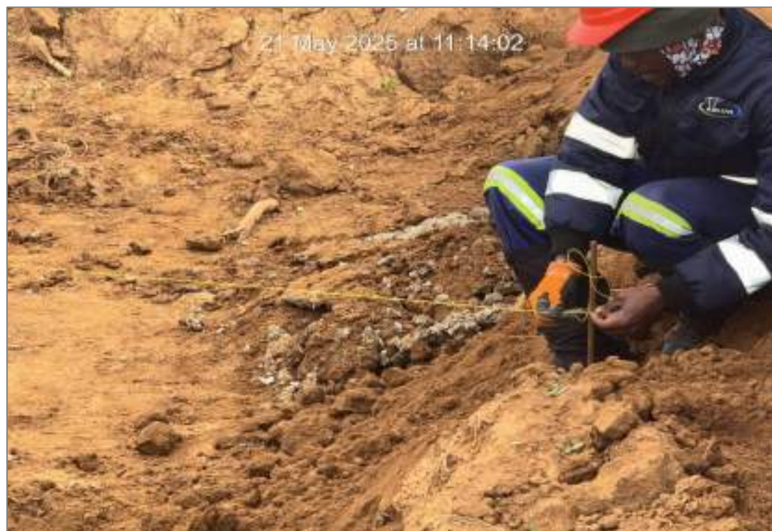
Figure 2: Concrete spillages that must be removed and not buried.
