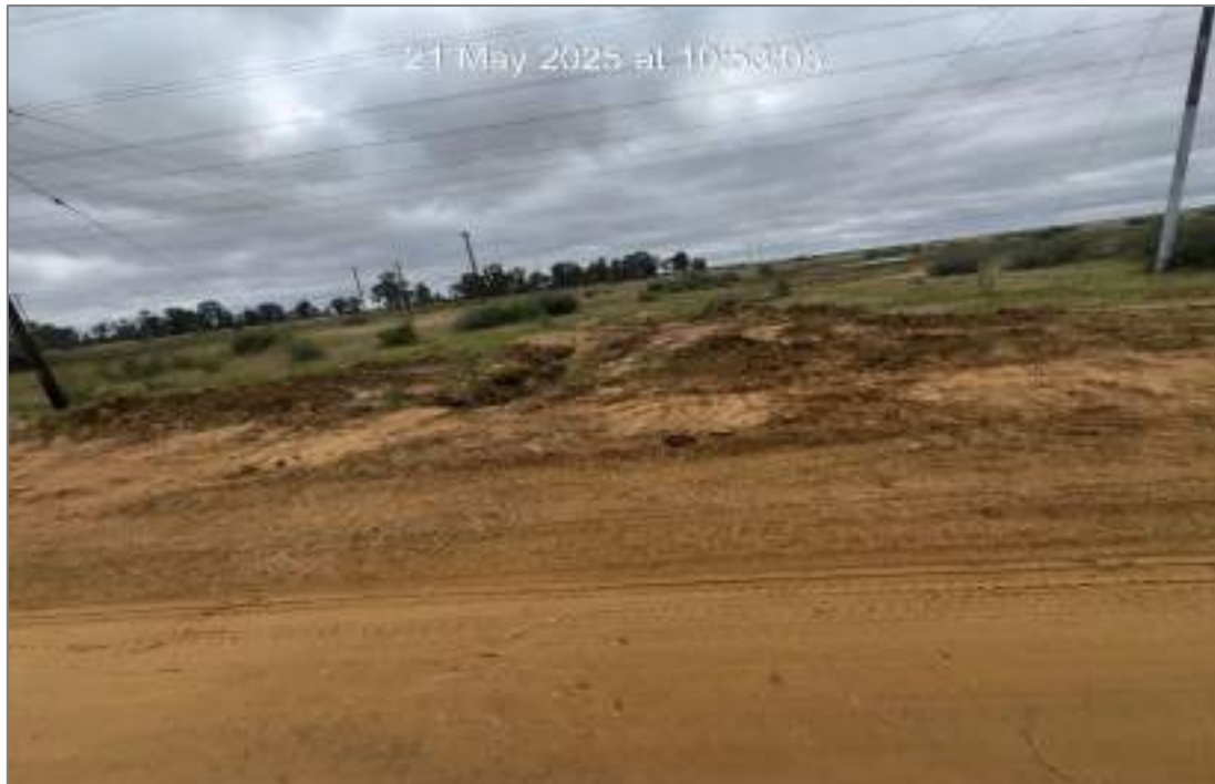
Figure 1: Erosion caused by pumped water.
