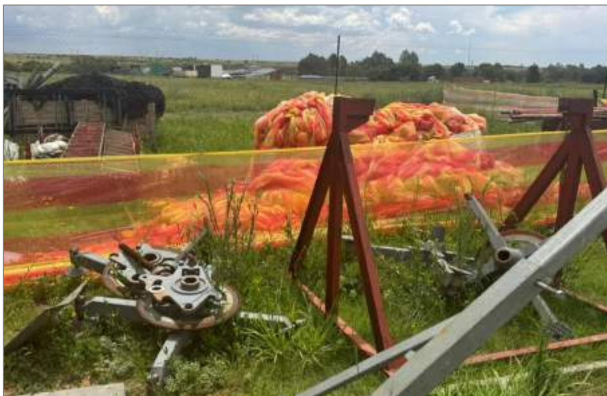
Figure 7: Torn barricading nets must be taken for recycling.
