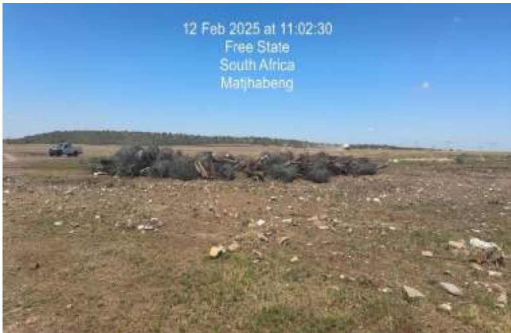
Figure 2: Removed fences must be reused or appropriately disposed of.
