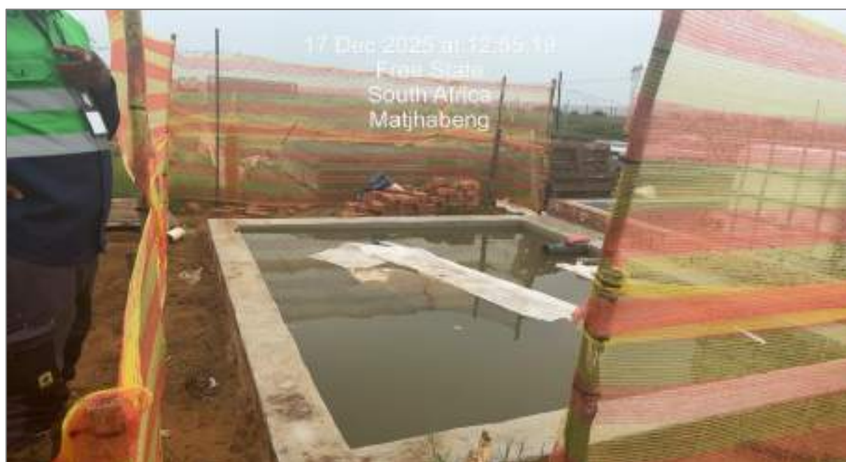
Figure 4: Overflowing sump at the waste area.
