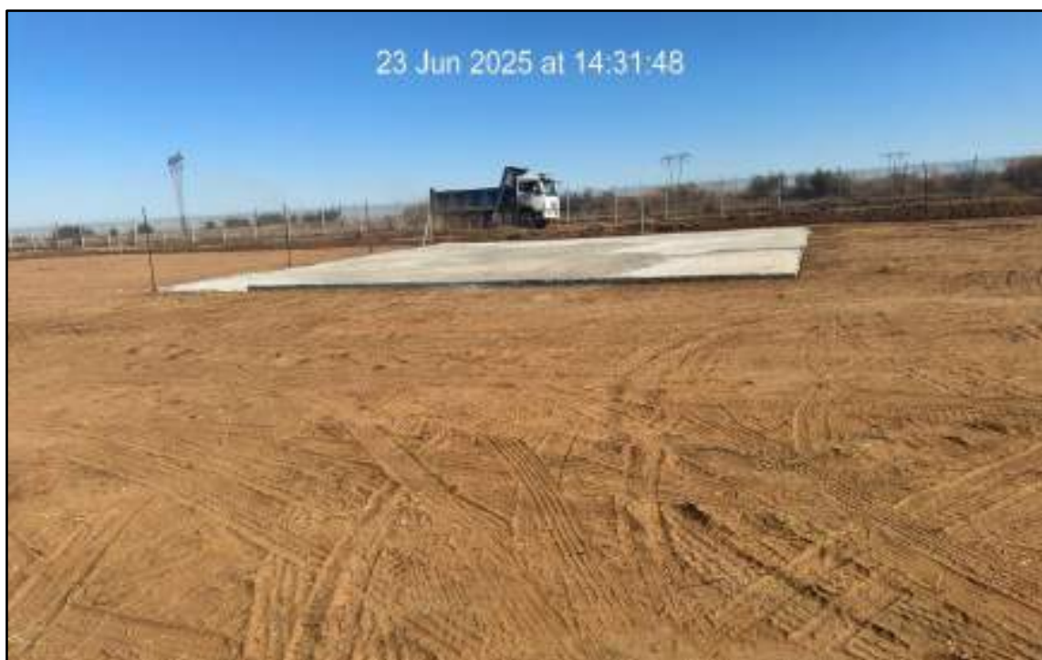
Figure 1: Incomplete concrete bund for the waste area.
