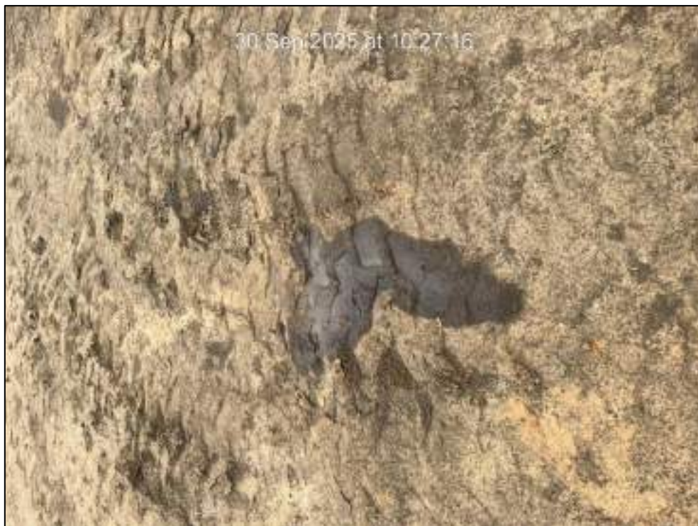
Figure 4: Small oil spillage.
