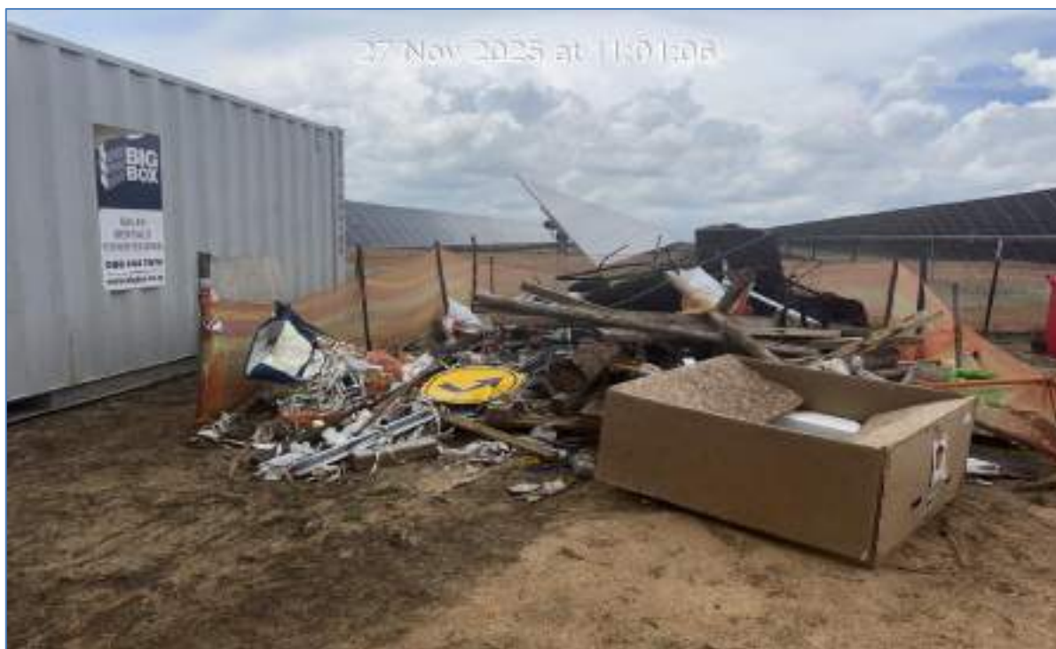
Figure 3: Poor waste management practices
