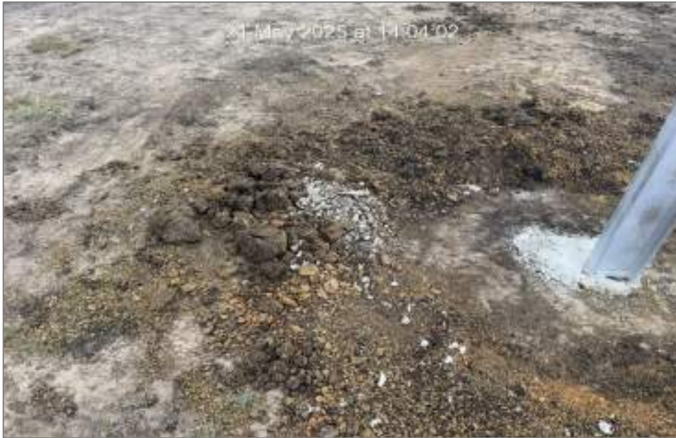
Figure 3: Concrete spillages that must be removed and not buried.
