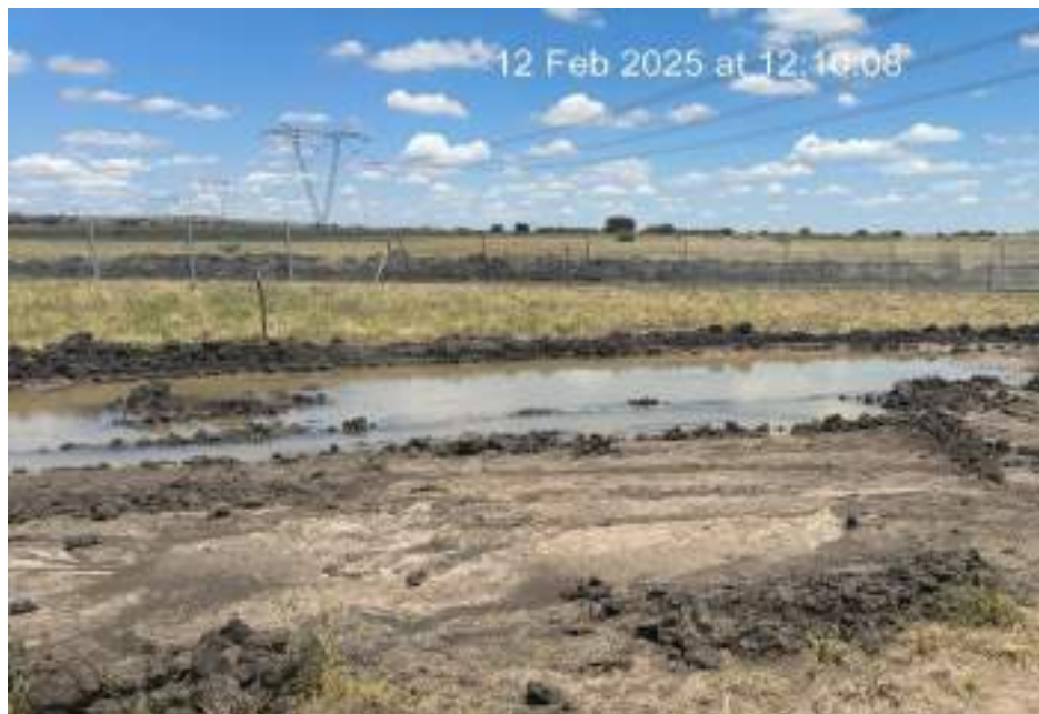
Figure 6: Water ponding onsite
