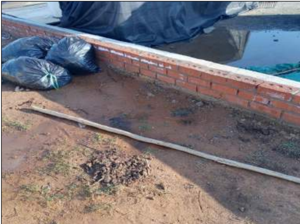
Figure 12: Leaking waste bund.
