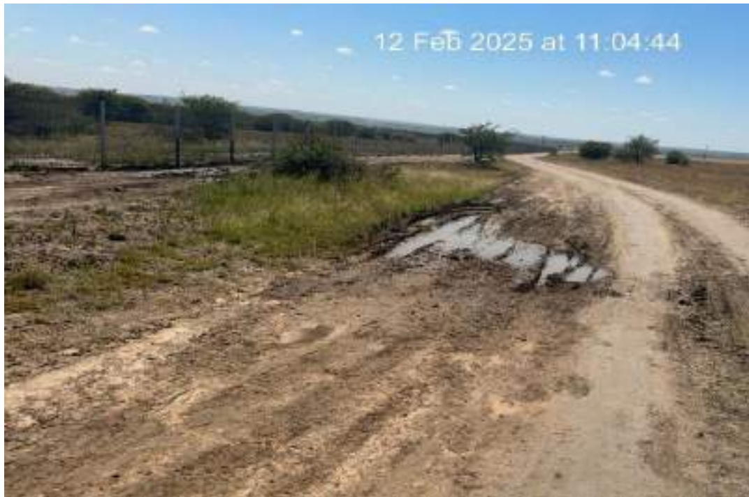
Figure 3: Access roads requiring regrading.
