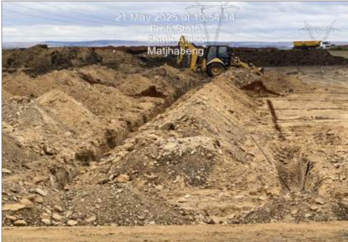
Figure 5: Excavation that must be barricaded.
