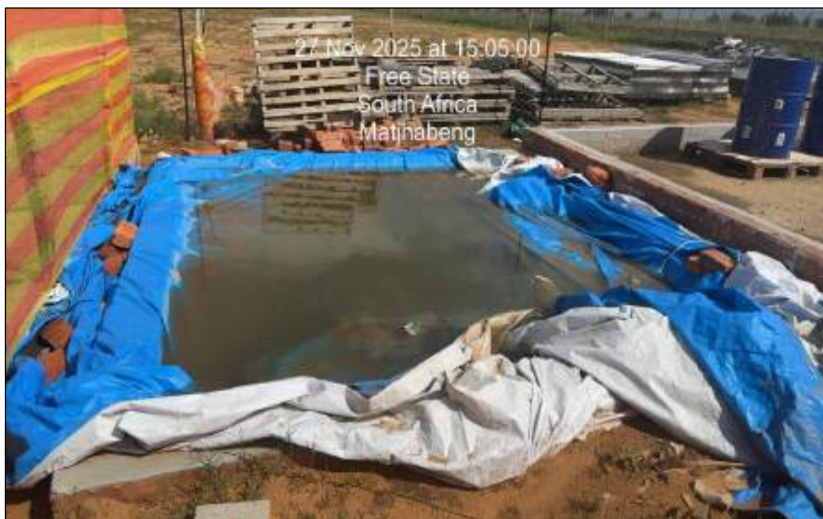
Figure 4: Overflowing sump at the waste area
