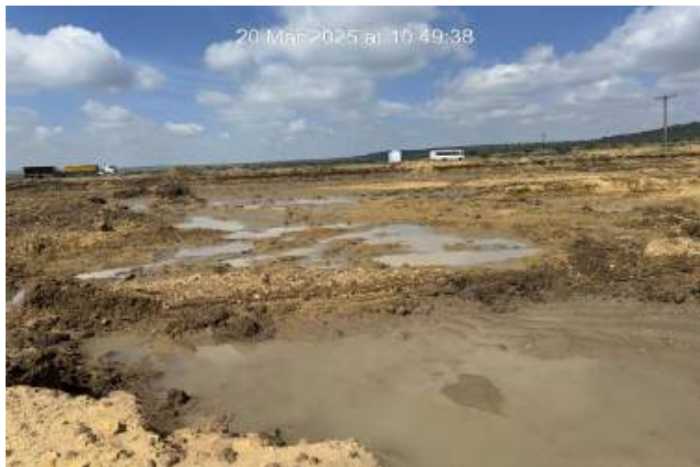
Figure 6: Water ponding onsite
