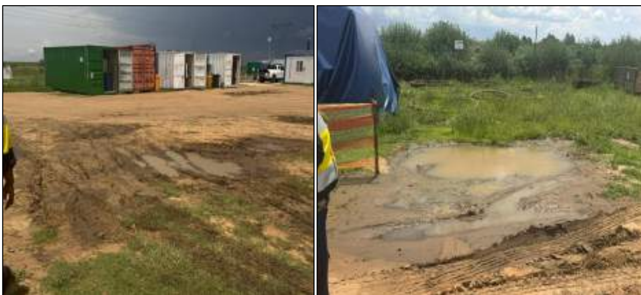
Figure 4: Water ponding at the laydown area
