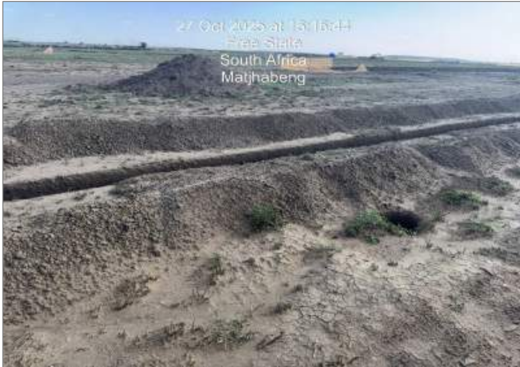
Figure 9: Open trenches left open unbarricaded.
