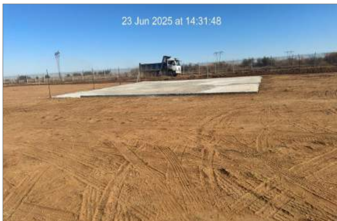
Figure 6: Incomplete concrete bund for the waste area
