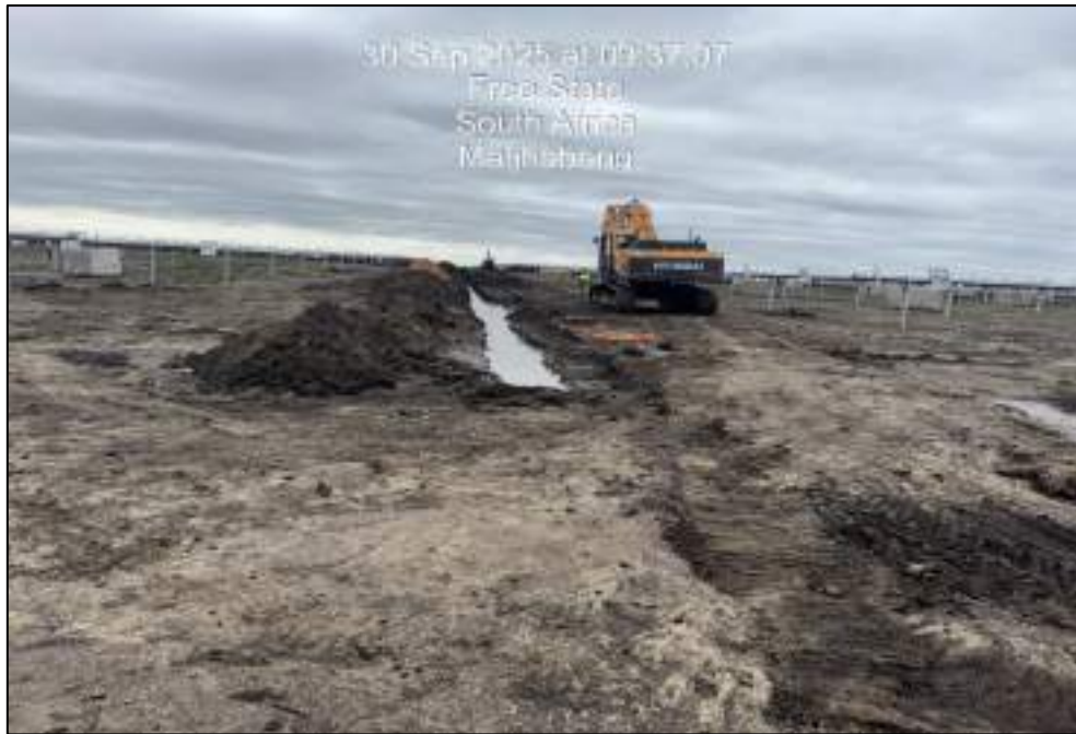
Figure 3: Unbaricaded trenches with water.
