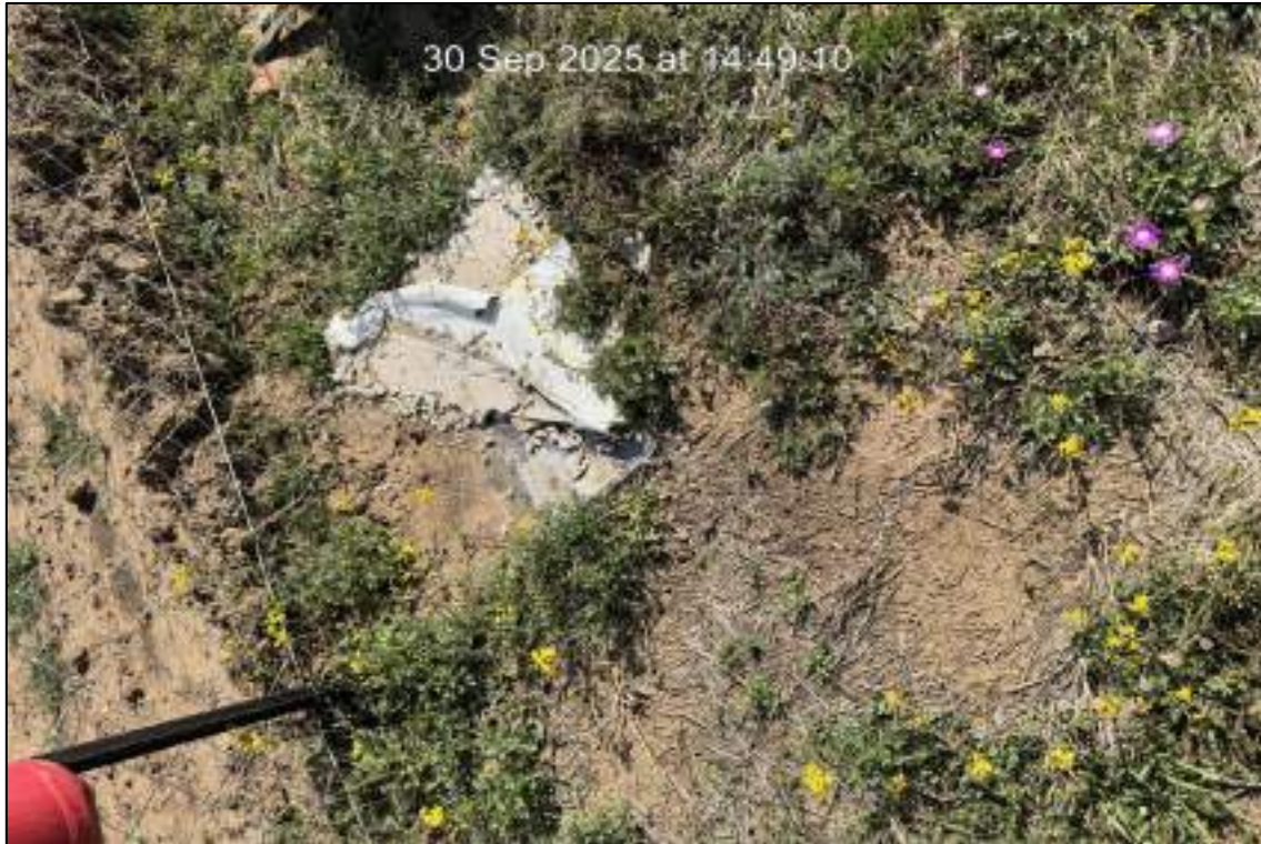
Figure 7: Concrete must be disposed correctly.
