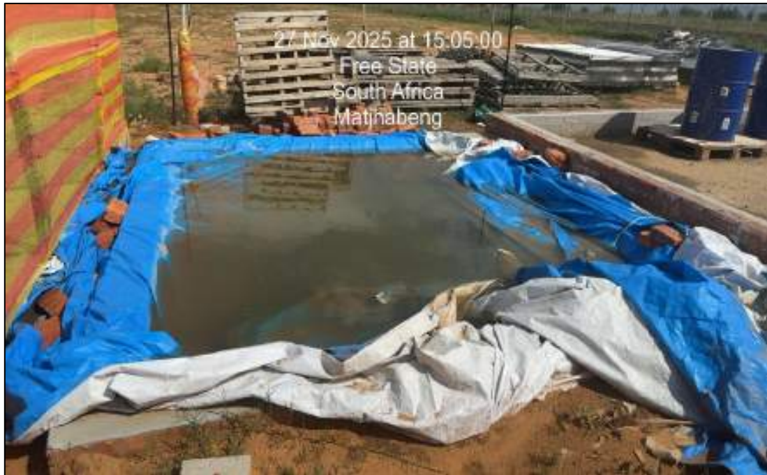
Figure 5: Overflowing sump at the waste area.
