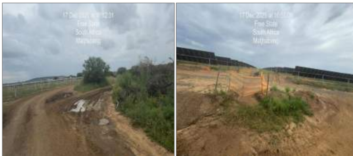
Figure 7: Damage to the road caused rainwater.
