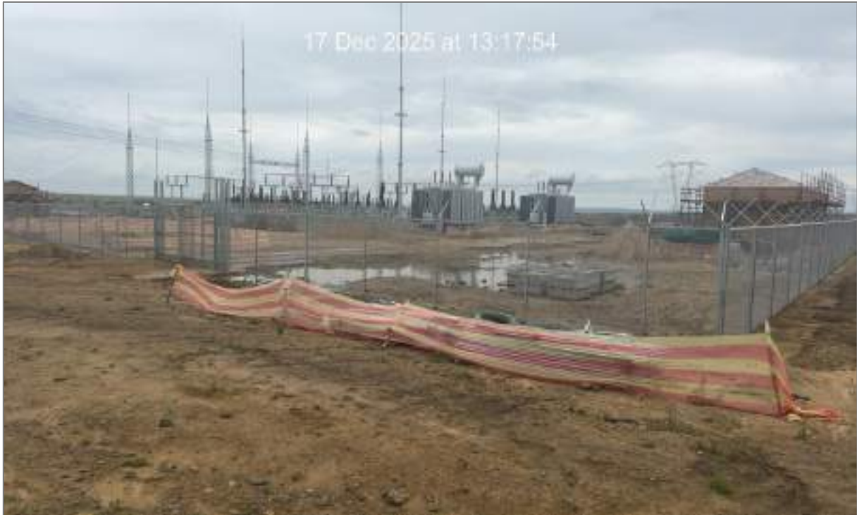
Figure 1: Water ponding at the substation area.
