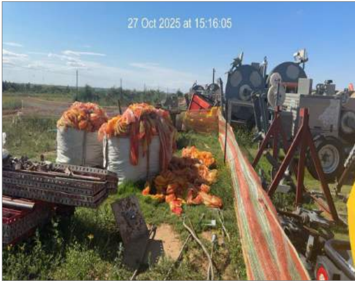
Figure 3: Torn barricade must be recycled.
