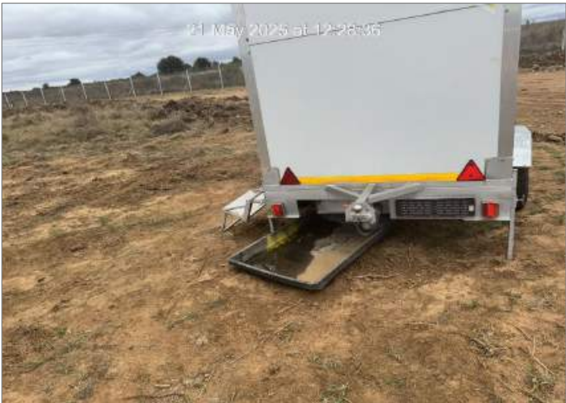
Figure 4: Drip tray provided for on the chemical toilet.
