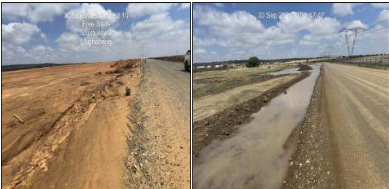
Figure 2: Sign of Erosion and water ponding onsite.
