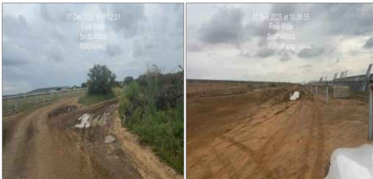
Figure 1: Condition of some portions of the access roads.
