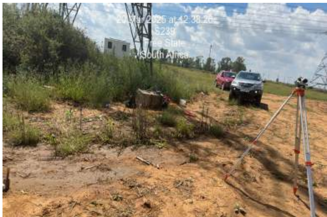
Figure 10: A Shaded area must be provided for people working on the powerline
