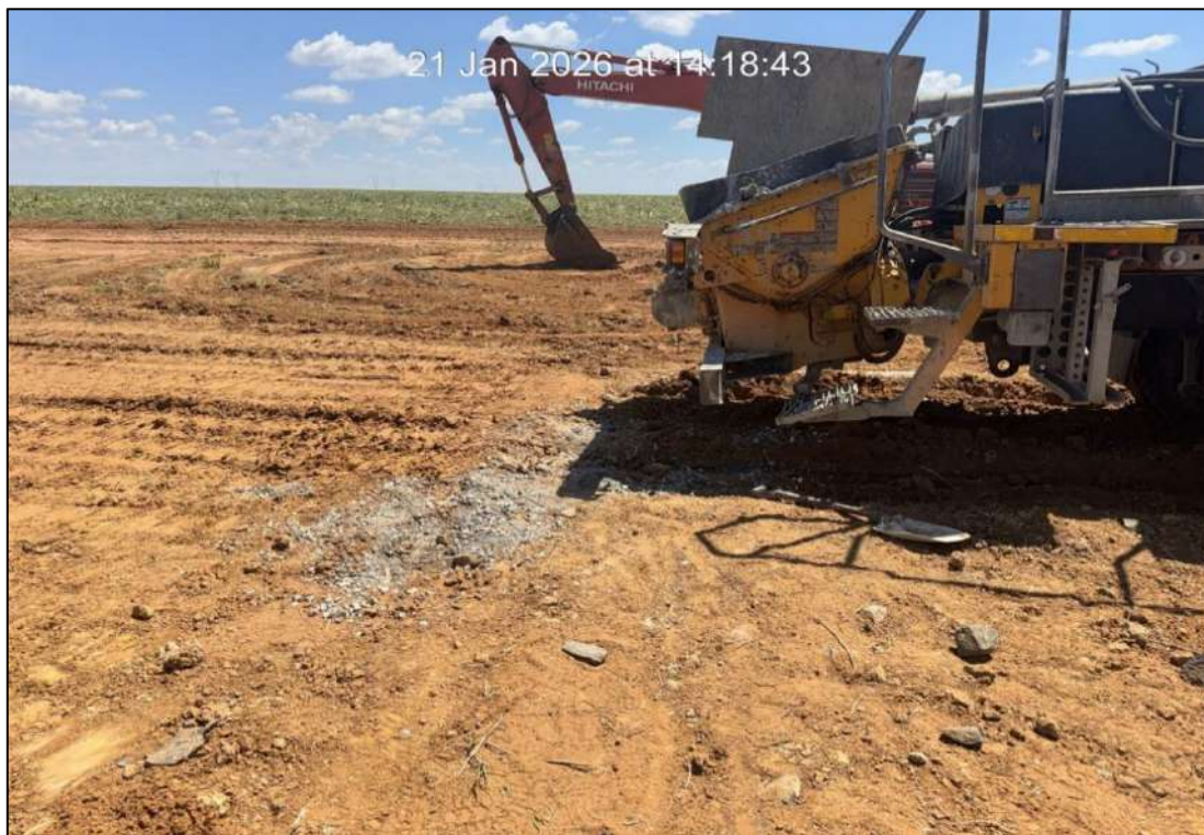
Figure 4: Spilled concrete must be removed before the end of the day.
