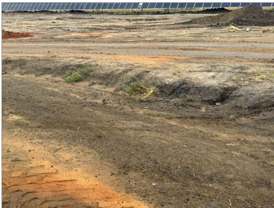
Figure 1: Condition of the access roads.
