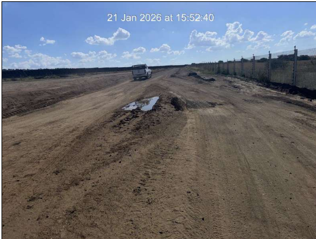
Figure 1: Condition of the access roads.
