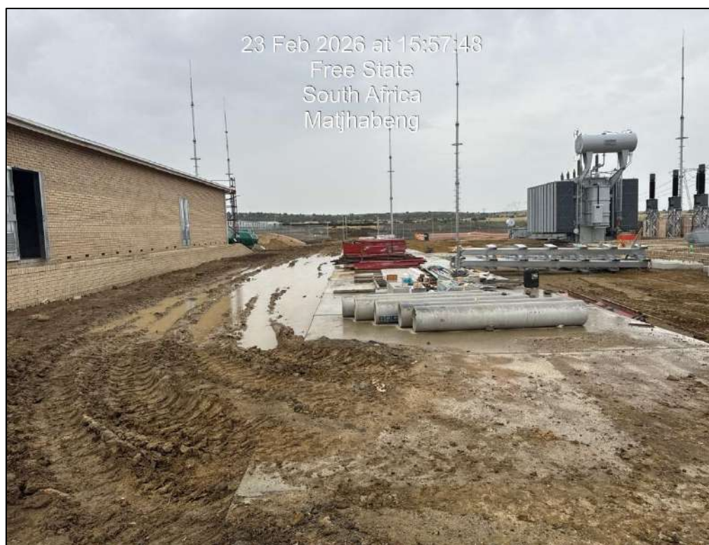
Figure 2: Water ponding and mud at the switching station
