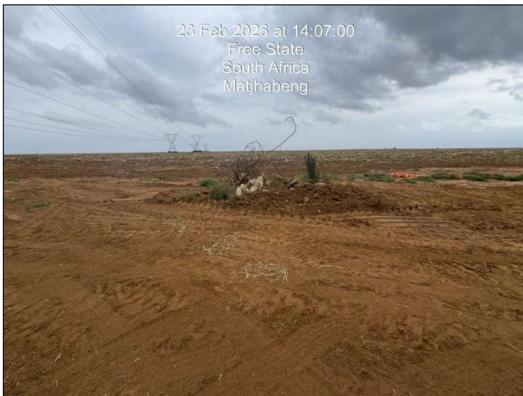
Figure 7: Rubble along the line.
