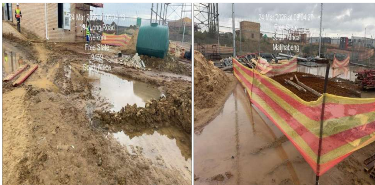
Figure 3: Water ponding and mud at the switching station
