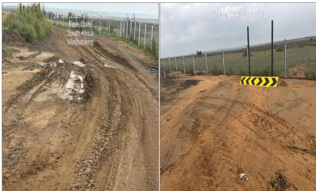
Figure 1: Condition of the access roads.
