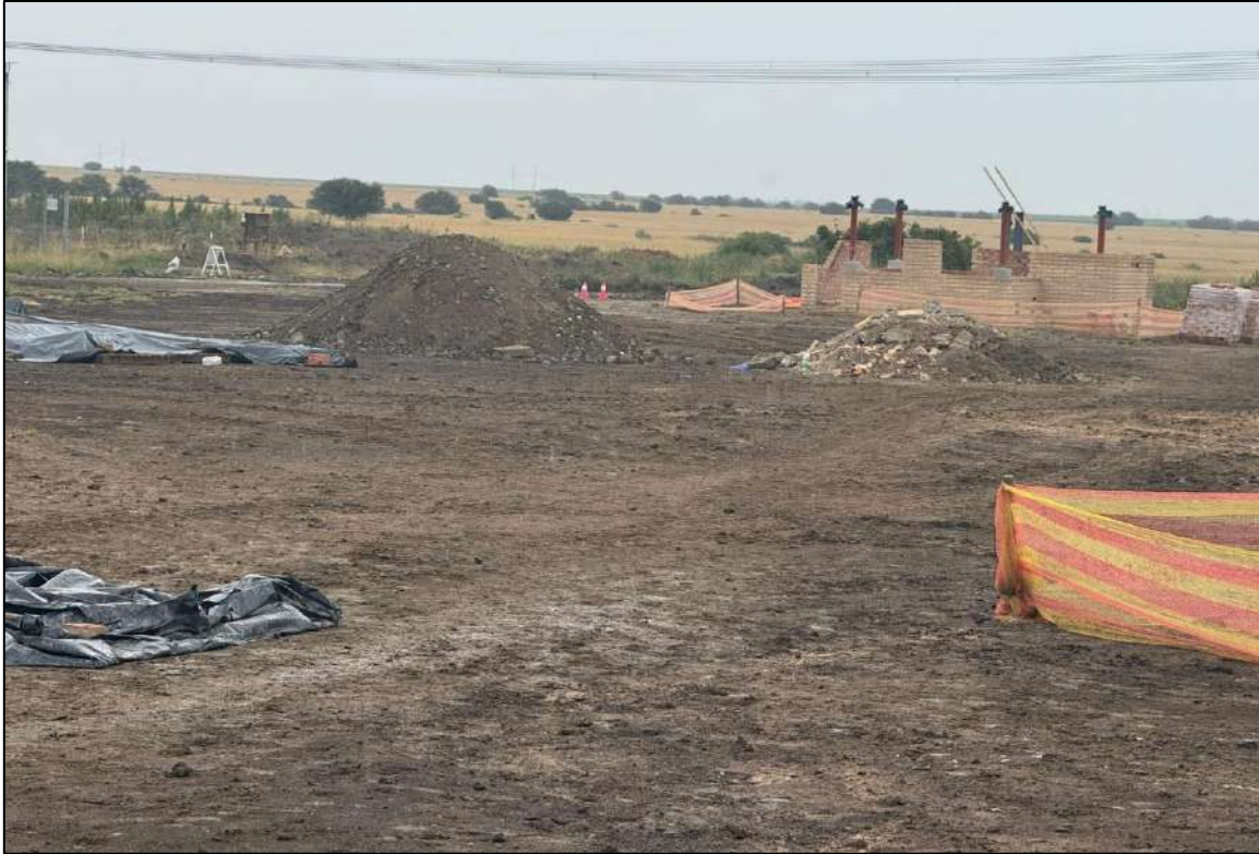
Figure 3: Construction Rubble at the switching station.
