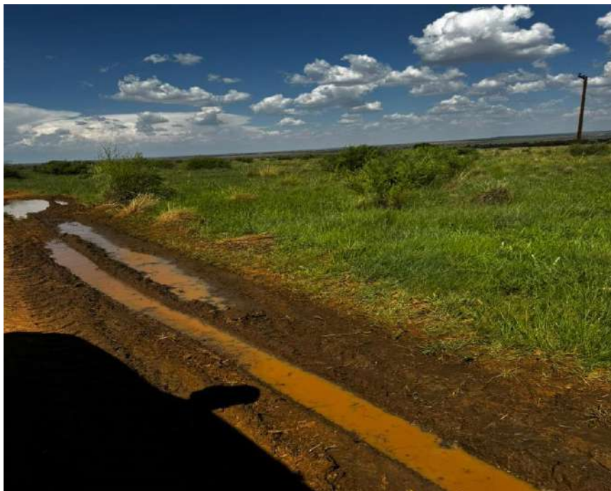
Figure 5: Water ponding on the access roads
