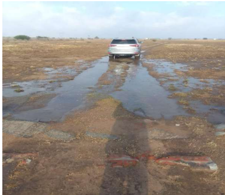
Figure 4: Water ponding on the access roads
