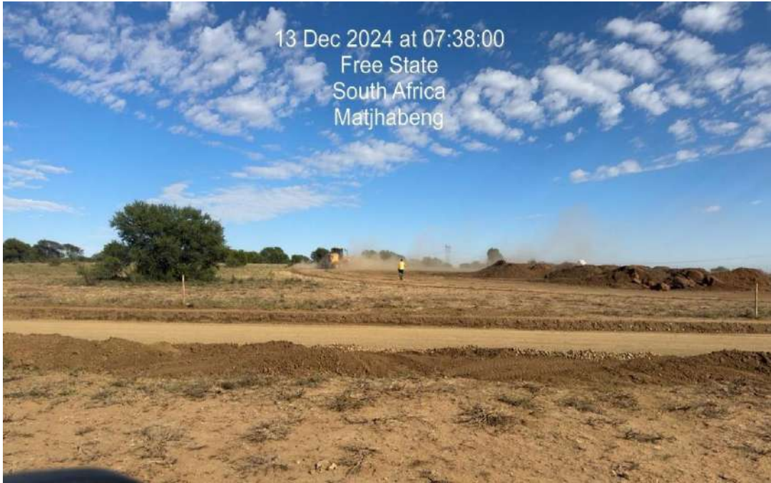
Figure 1: Excessive dust being generated.
