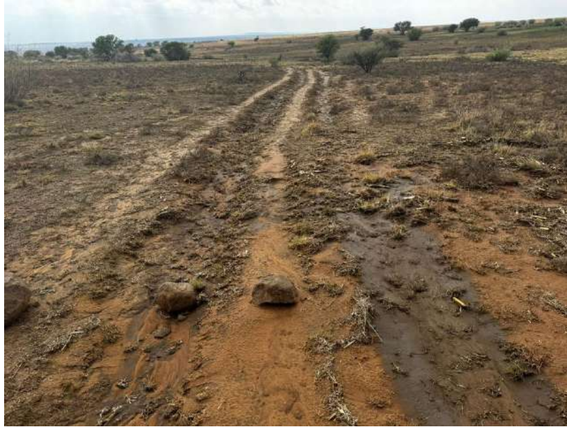
Figure 1: Erosion on the access roads
