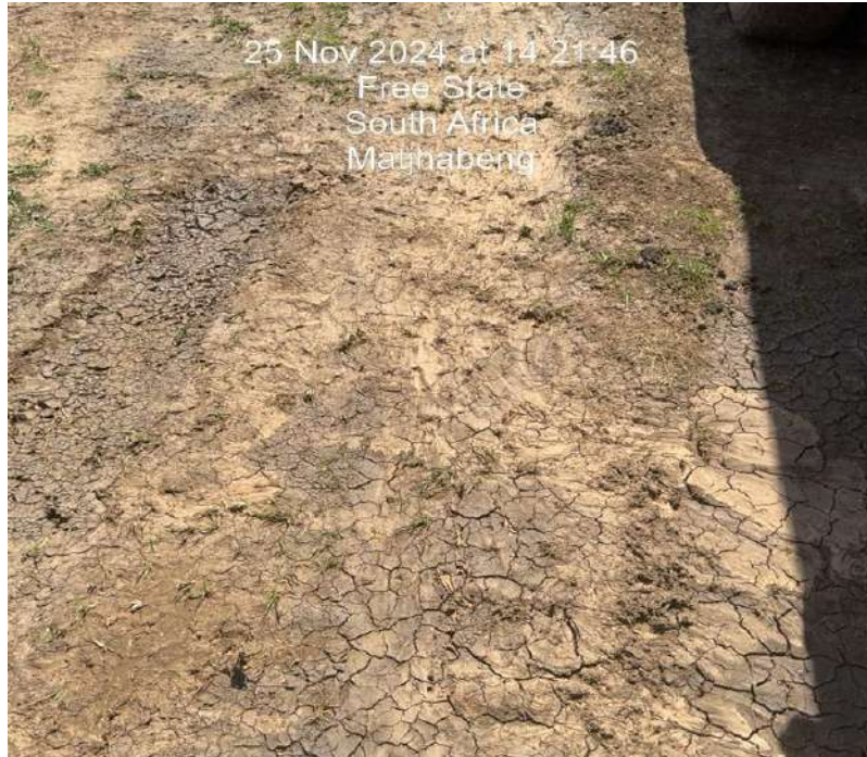
Figure 4: Erosion on the access roads
