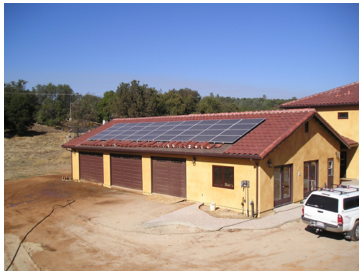
Static solar photo-voltaic system needs 50% more panels
