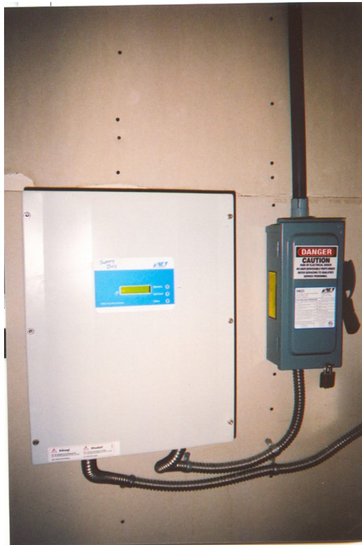
A simple power inverter for a grid-tie photovoltaic system
