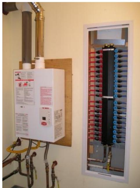
This is an example of a Bosch Aquastar on-demand water heater combined with a Vanguard manablock manifold plumbing system. this is the most energy efficient way to heat and distribute water (photo courtesy hurst construction)
