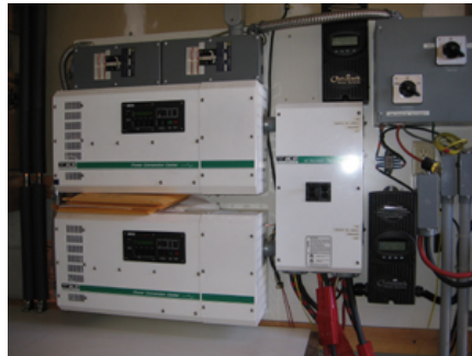
Power inverters and control room this is a grid tie system meaning we are hooked up to the power grid and we can sell power back to them! (photo courtesy Sunfire research.)
