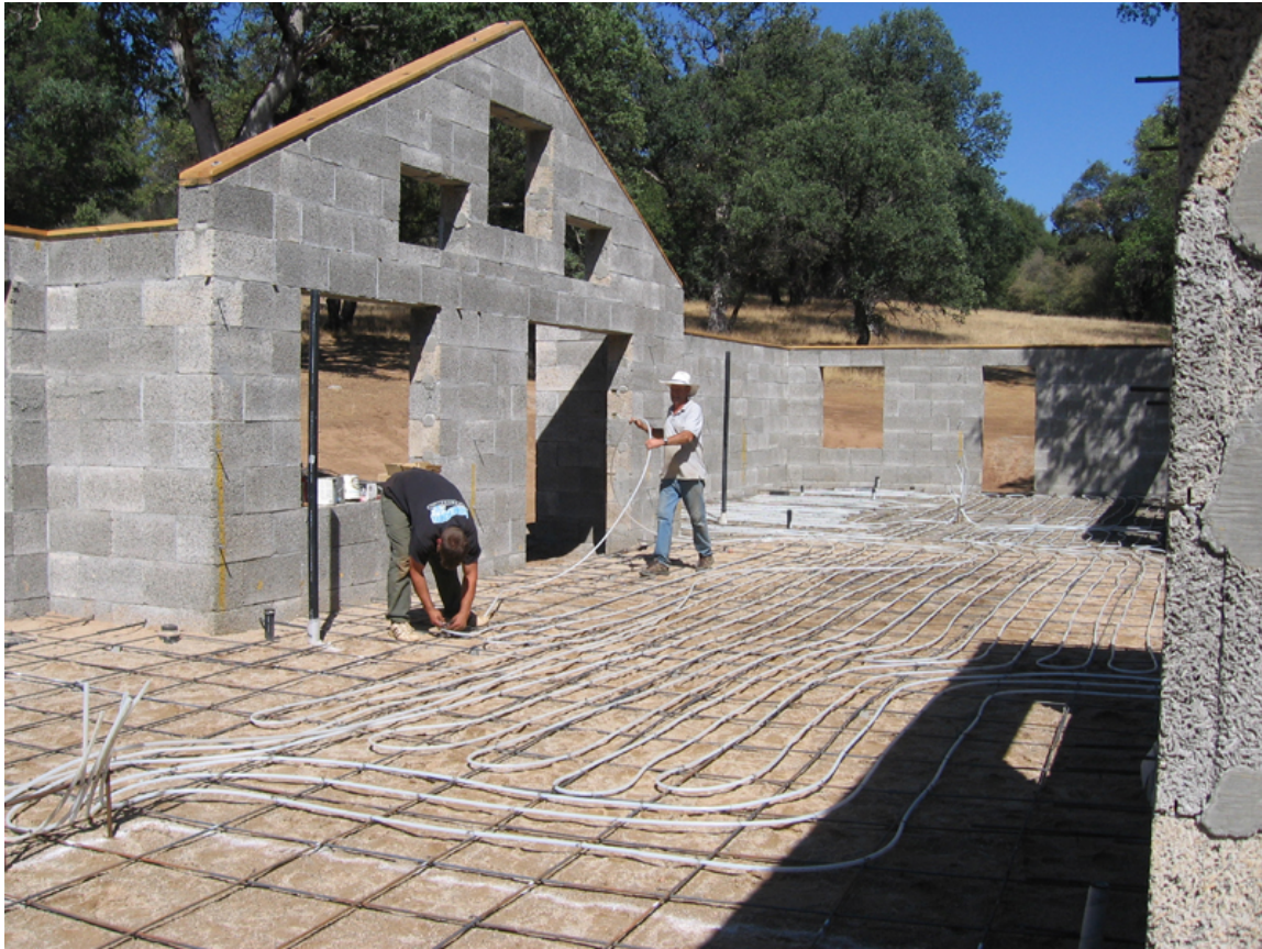
The Hurst construction crew installing the radiant heating system in a passive solar Durisol home.
