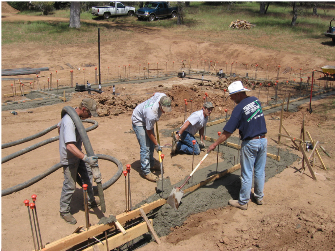
Fill the footings with concrete and level to the bottom of the screed board.
