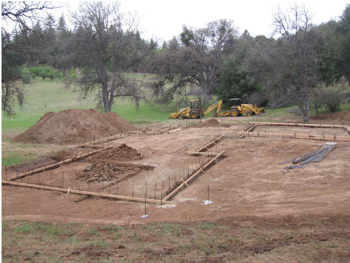
The footings have been dug and the re bar and the screed board is in place and we are ready to pour the concrete.
