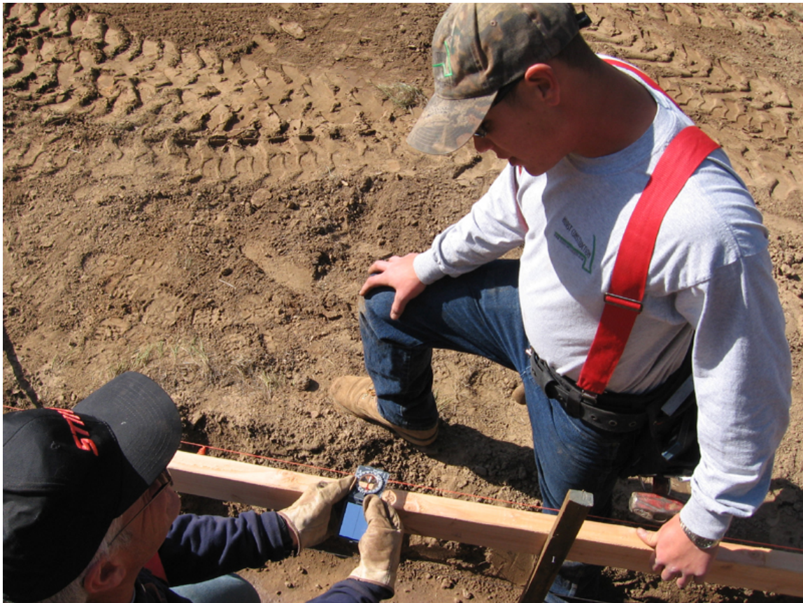
The Hurst construction crew checks the building footings for proper solar orientation with a compass.
