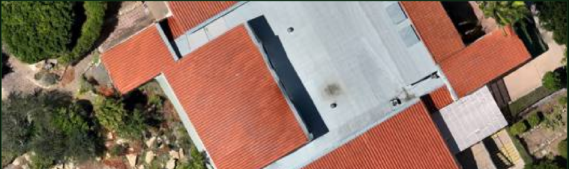
WEATHERING & DEBRIS DISCOLORATION
