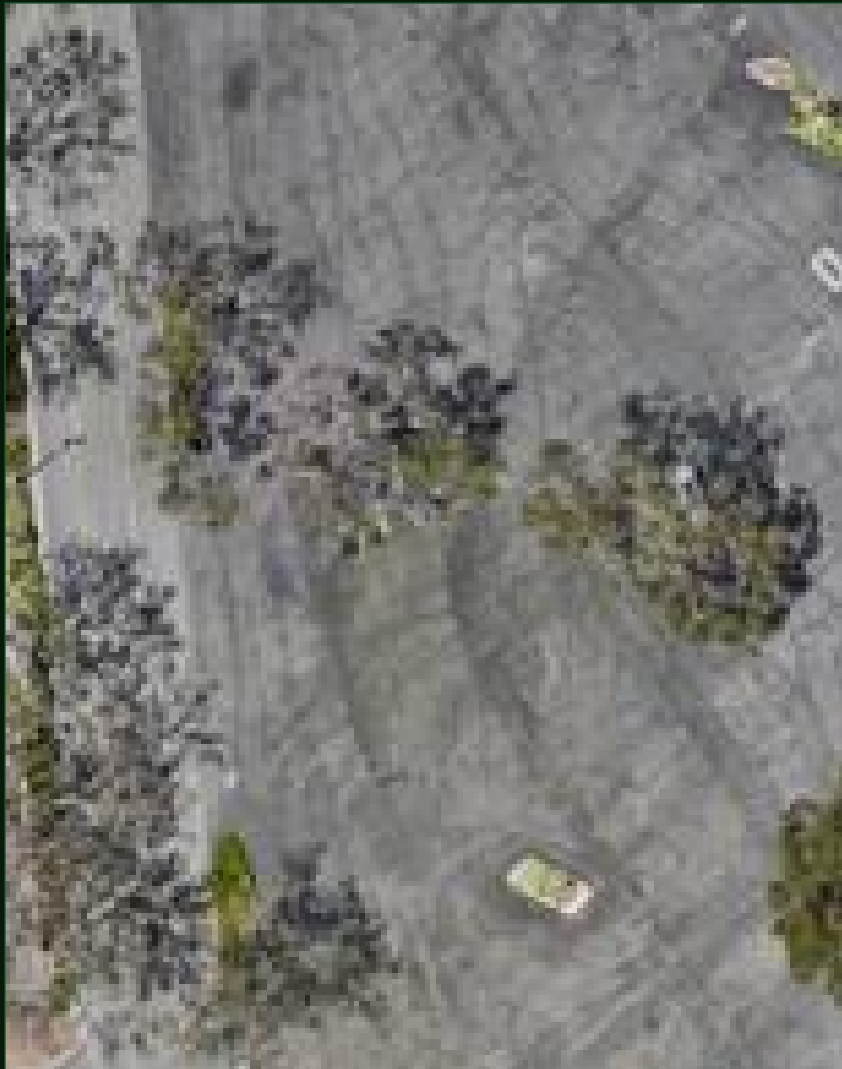
PARKING FIELD — SURFACE WEAR
