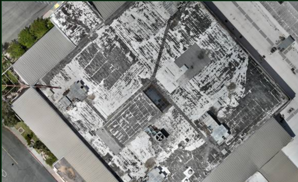
WEATHERING & DEBRIS DISCOLORATION
