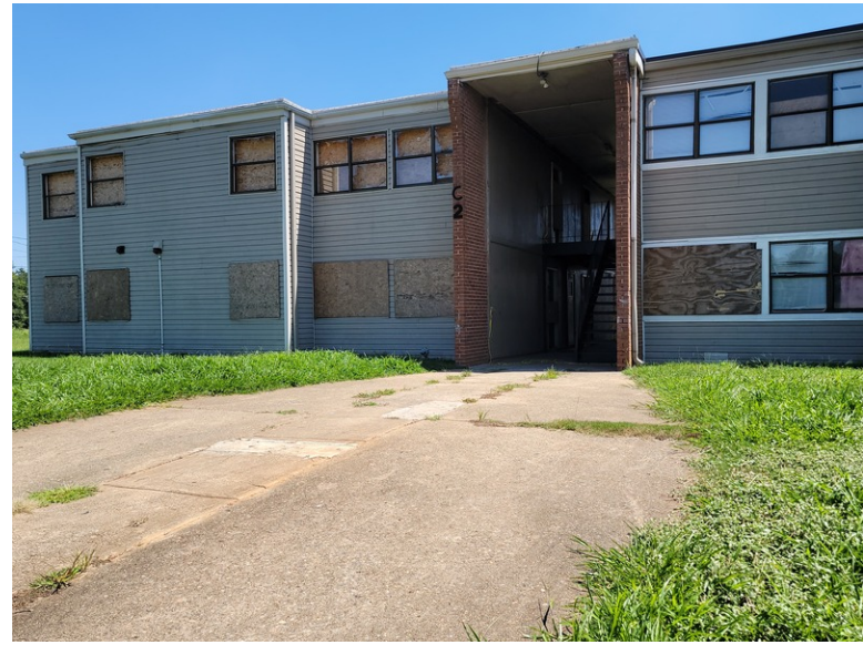
Picture #6: Boarded up Bldg C2 due to fire damage
