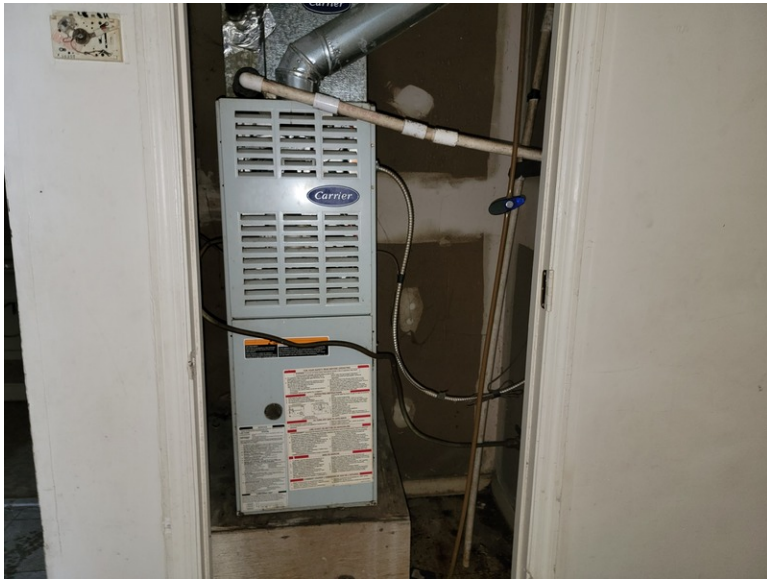
Picture #13: Natural gas-fired furnace in an apartment
