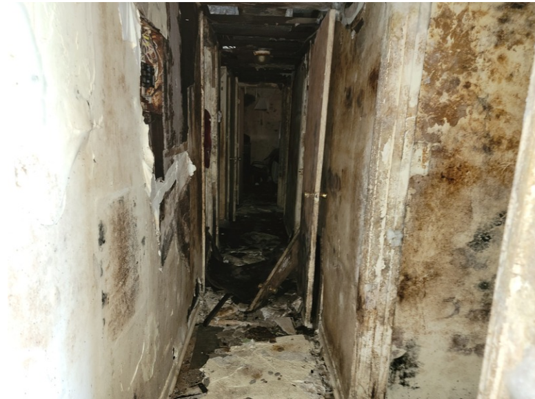
Picture #24: Mold growth in a down unit
