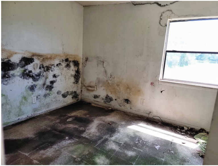
Picture #29: Mold growth in a down unit
