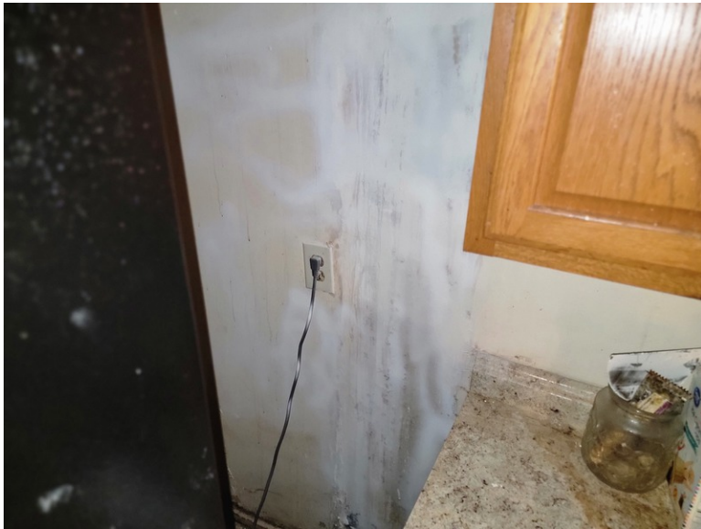
Picture #27: Mold growth in an occupied unit
