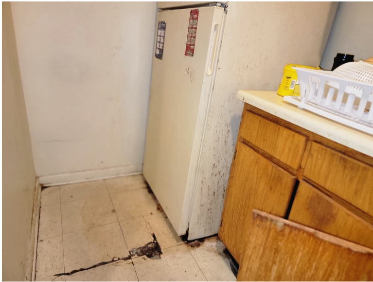
Picture #17: Damaged SAC vinyl floor tiles in an occupied unit
