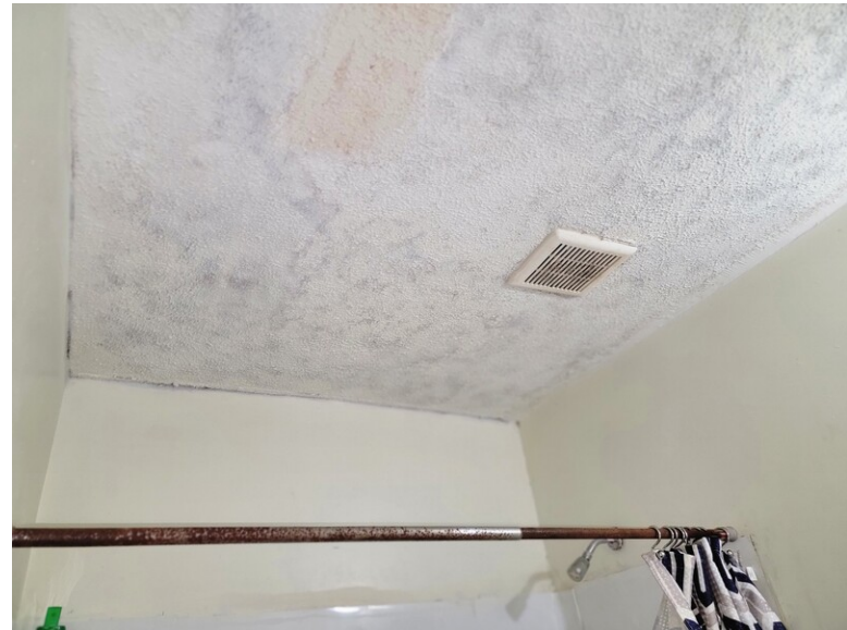
Picture #28: Mold growth in an occupied unit
