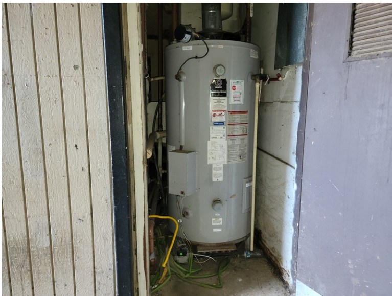
Picture #15: Natural gas-fired water heater in an apartment
