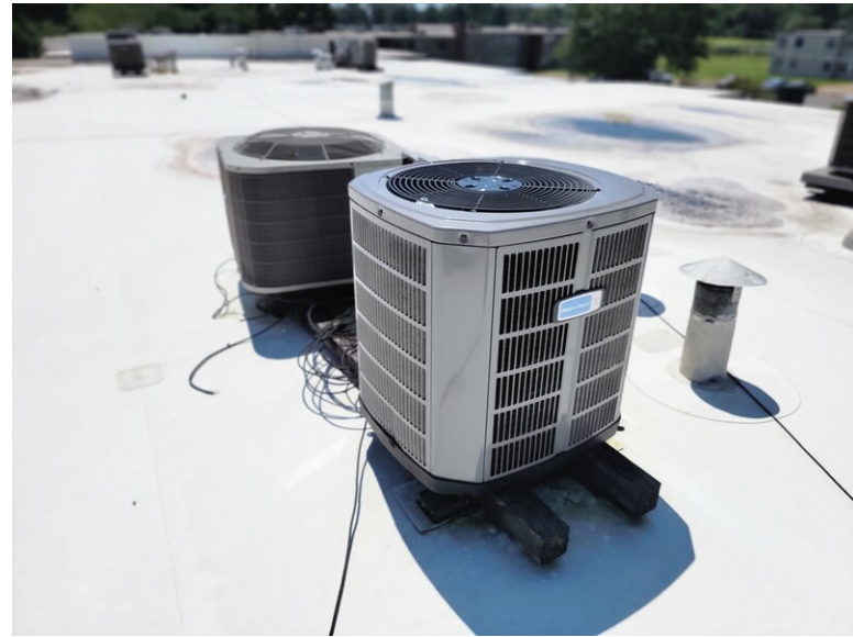
Picture #14: Condenser units on a roof
