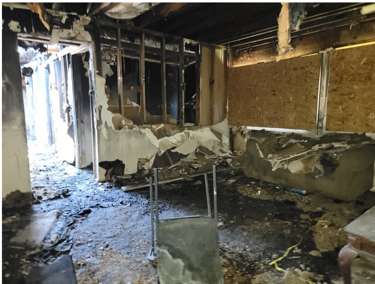
Picture #19: Damaged painted surfaces in a down unit
