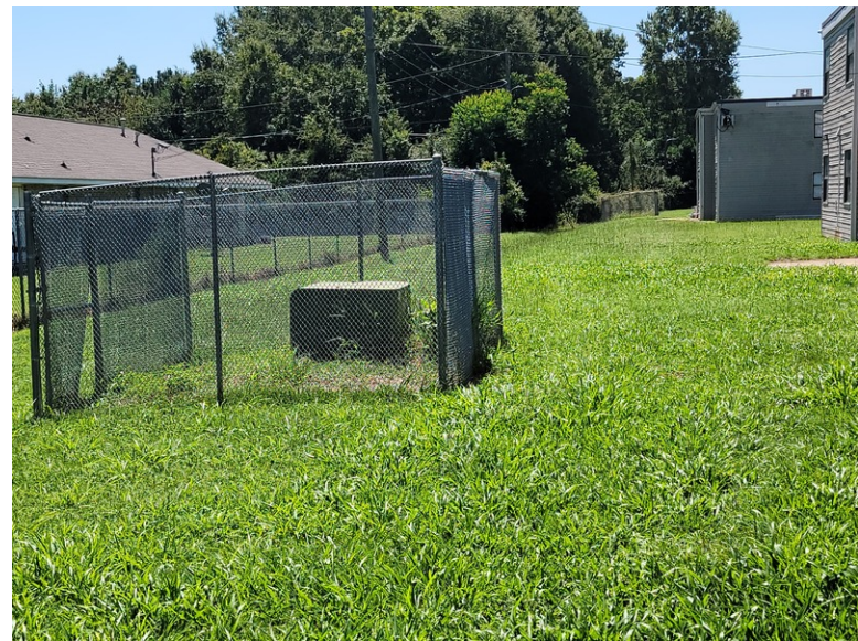
Picture #20: Utility-owned transformer
