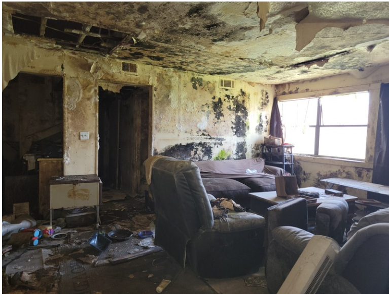
Picture #23: Mold growth in a down unit
