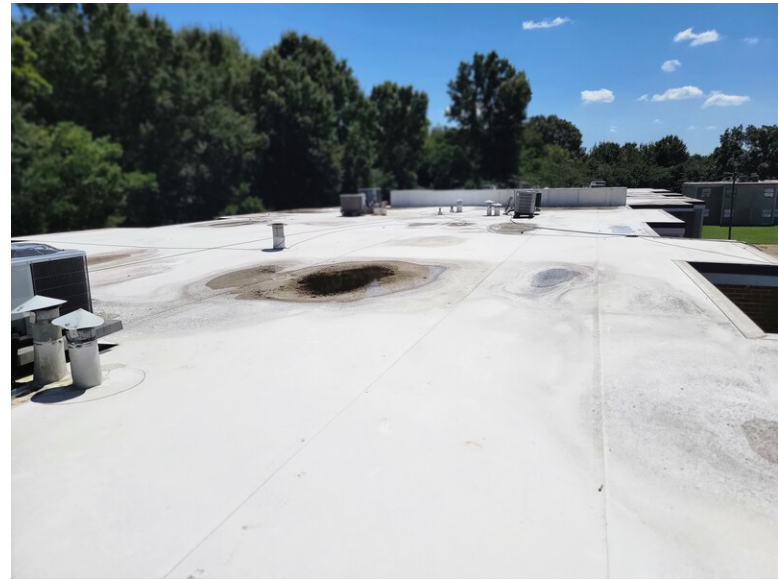
Picture #18: Non-friable SAC roofing materials
