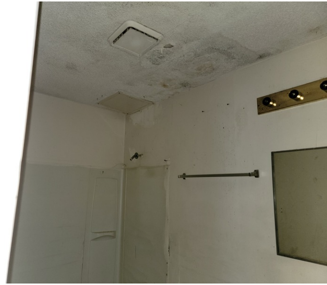
Picture #26: Mold growth in a vacant unit
