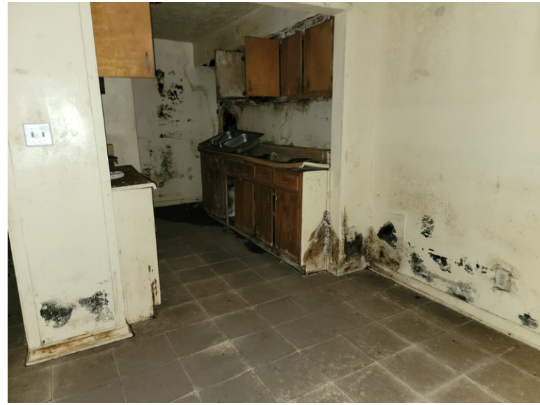
Picture #22: Mold growth in a down unit
