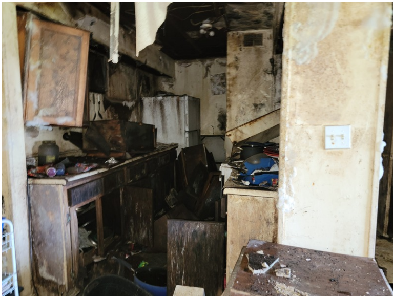
Picture #25: Mold growth in a down unit
