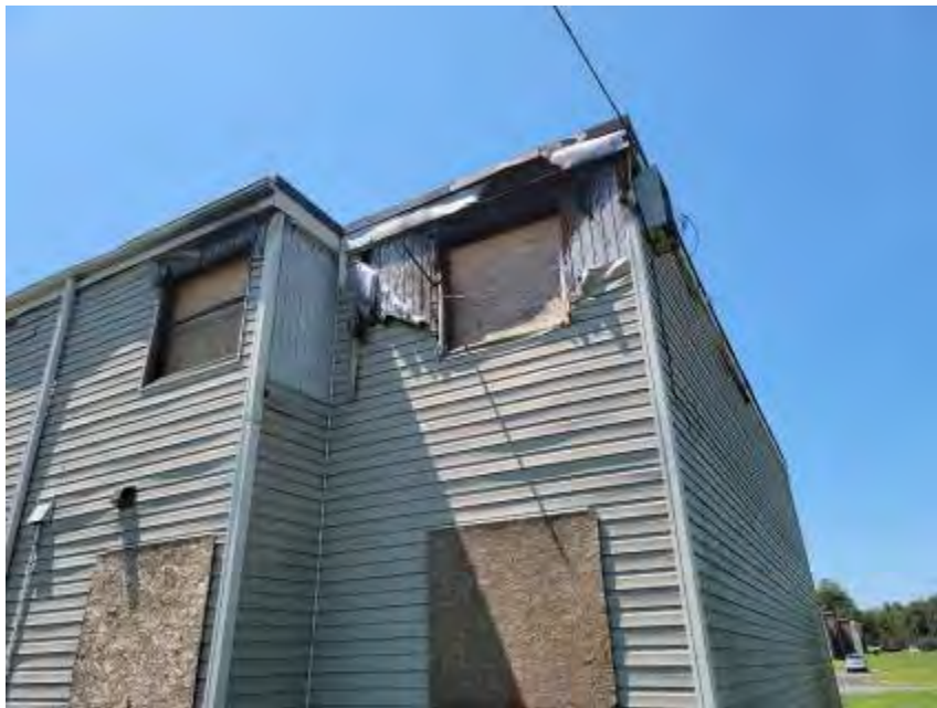
Picture #15: Damaged siding due to fire
