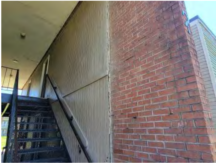
Picture #13: Siding that has open joint
