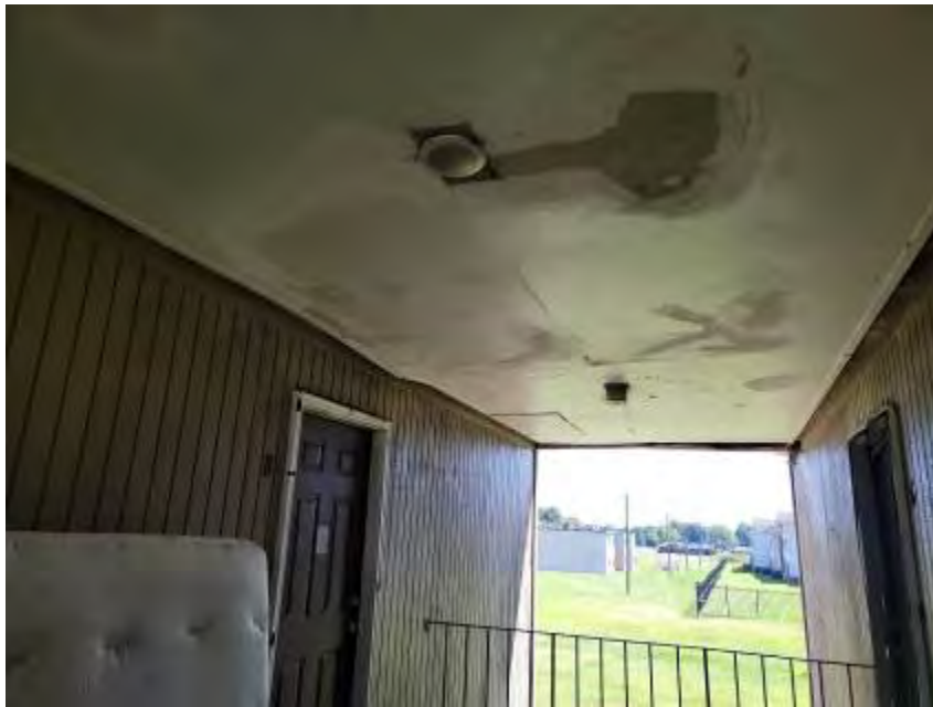
Picture #21: Damaged soffits in breezeways
