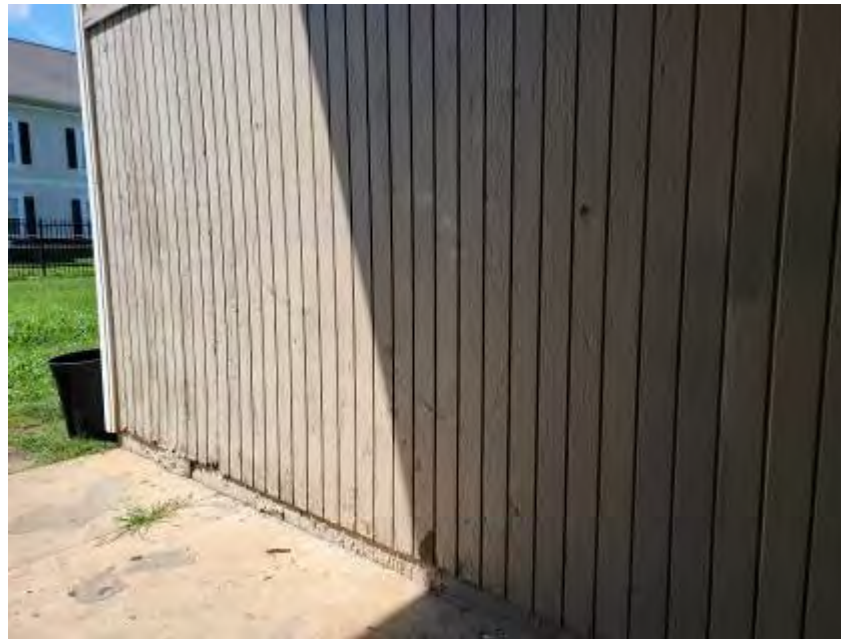
Picture #18: Damaged T1-11 siding
