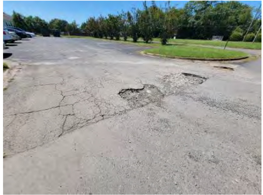
Picture #2: Potholes and damage on asphalt pavement
