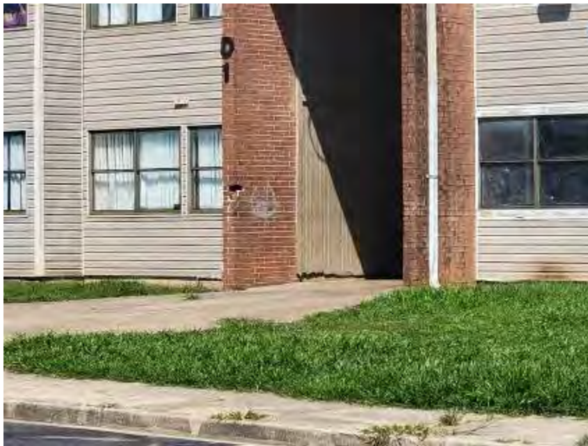
Picture #23: Damaged brick and graffiti – note the staining on the walls
