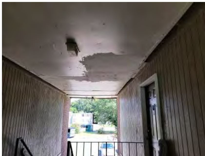
Picture #20: Damaged soffit in breezeways
