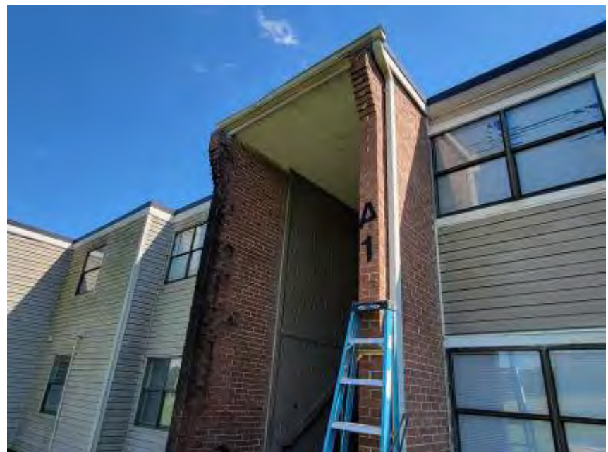
Picture #12: A typical breezeway entrance – note the staining on the walls (likely from leaking gutters)
