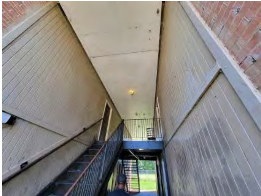
Picture #17: Graffiti that has not been properly removed – note the peeling paint on the railings
