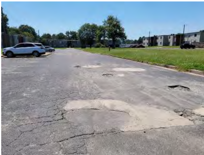
Picture #3: Potholes and damage on asphalt pavement
