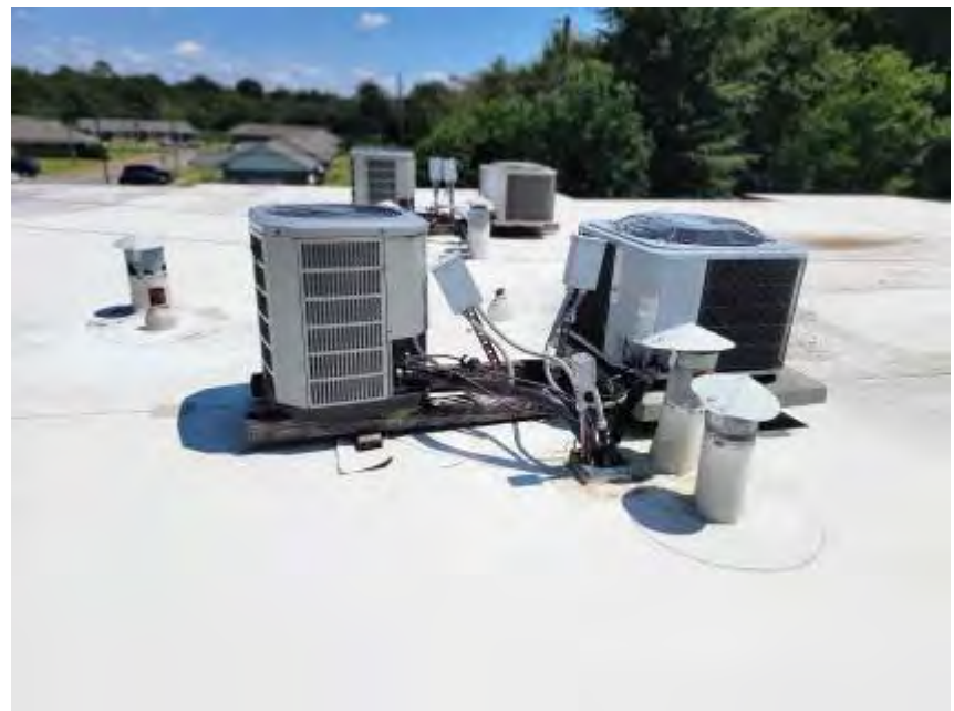
Picture #28: Typical condenser units
