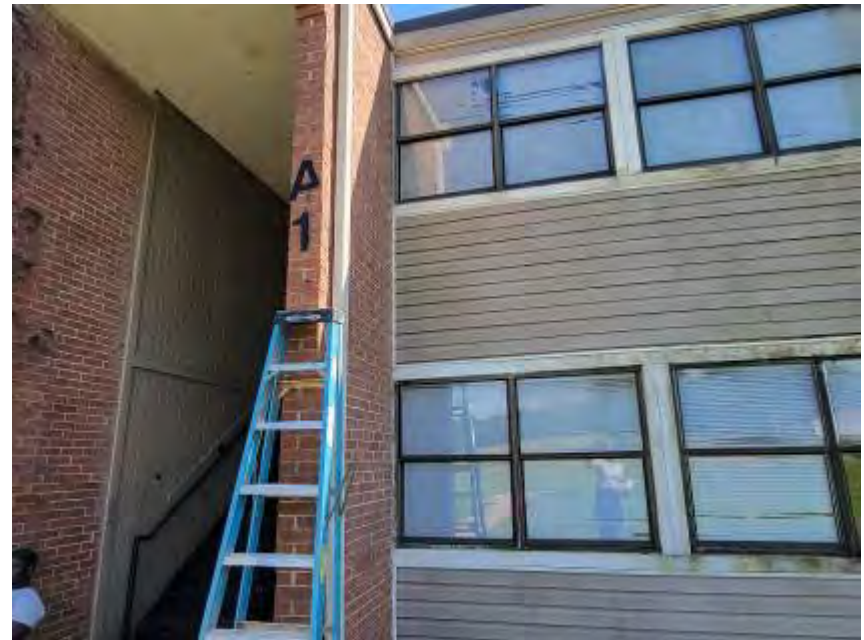
Picture #22: Mildew staining on the windows and facades
