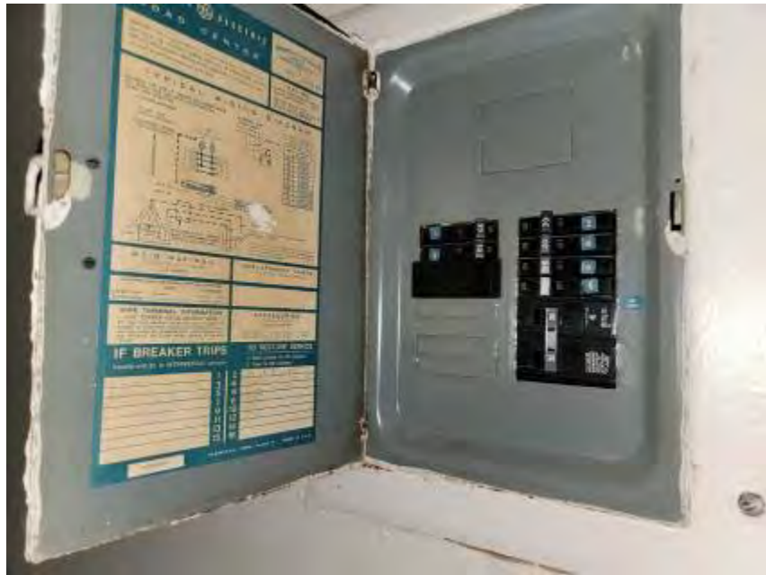
Picture #33: A typical apartment breaker panel
