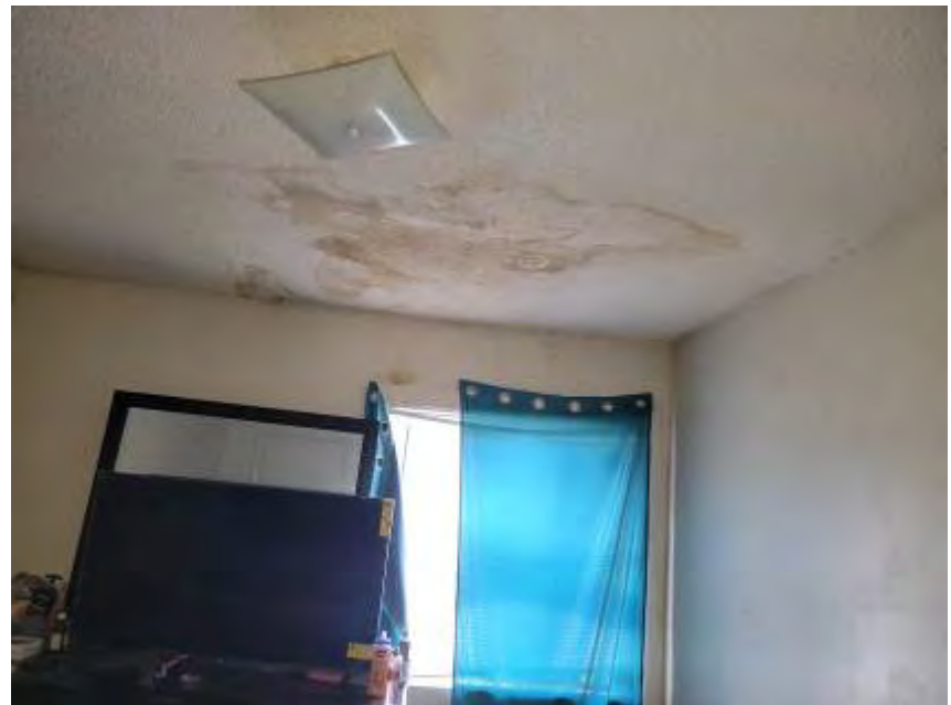
Picture #52: Unit F2-8 – likley an active roof leak
