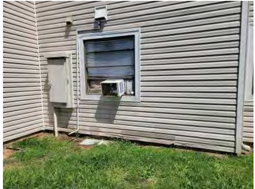
Picture #30: A typical window air conditioning unit
