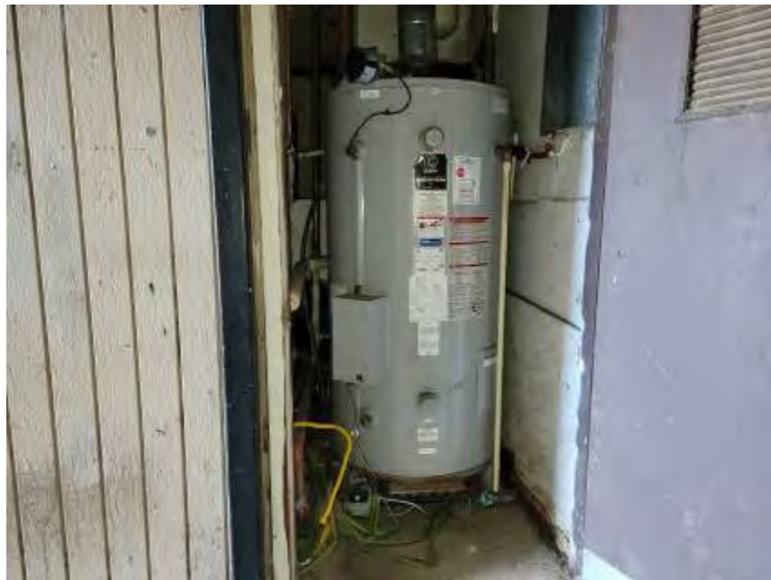
Picture #31: A typical water heater
