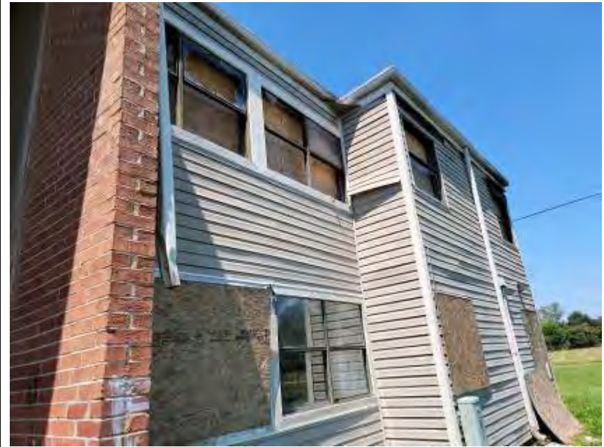
Picture #14: Fire damaged building
