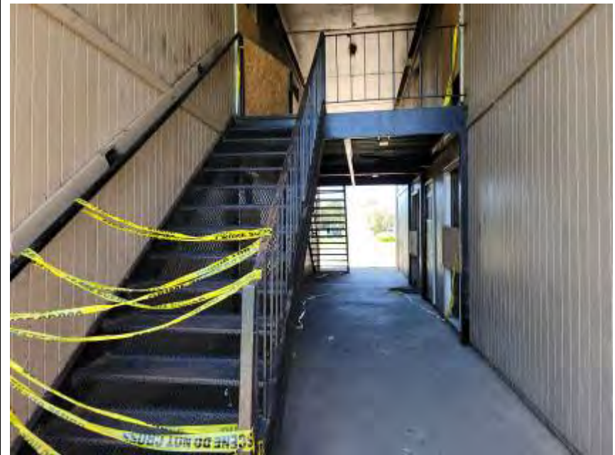
Picture #16: Breezeway and stairs (fire damaged building).
