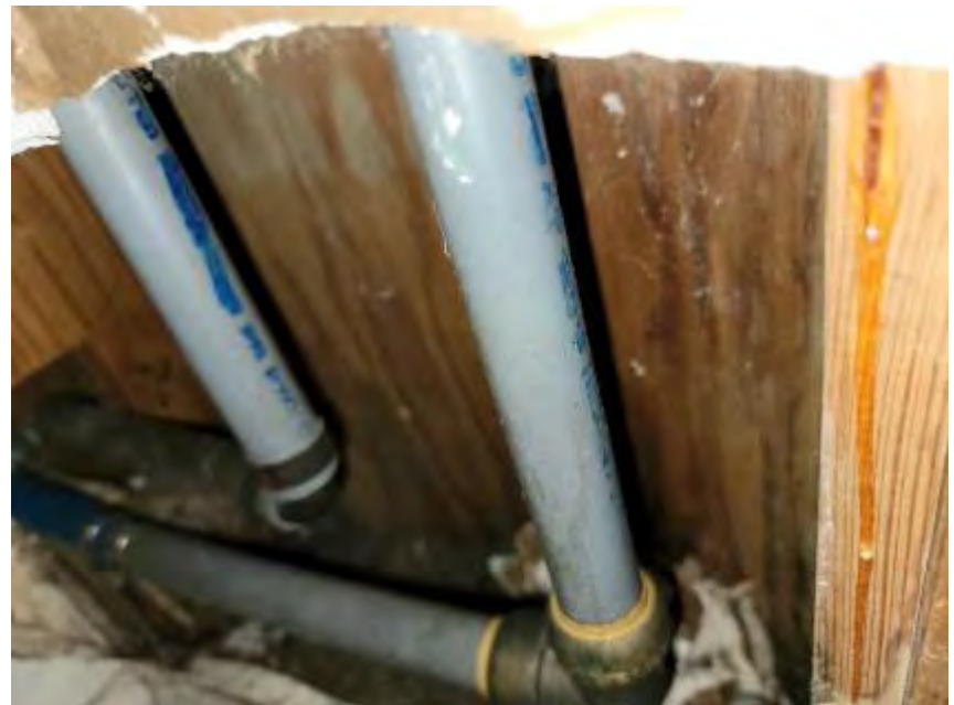
Picture #32: PB piping
