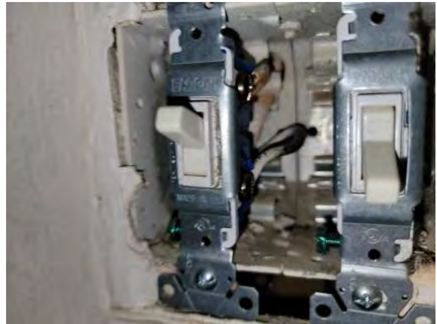
Picture #34: Copper branch wiring
