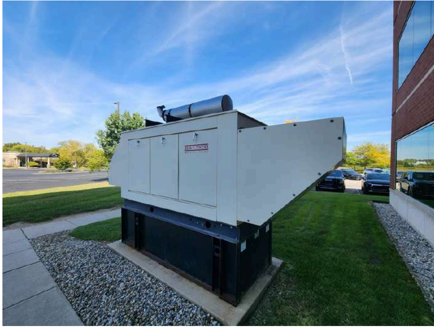
15. Tenant-owned generator at 8520
