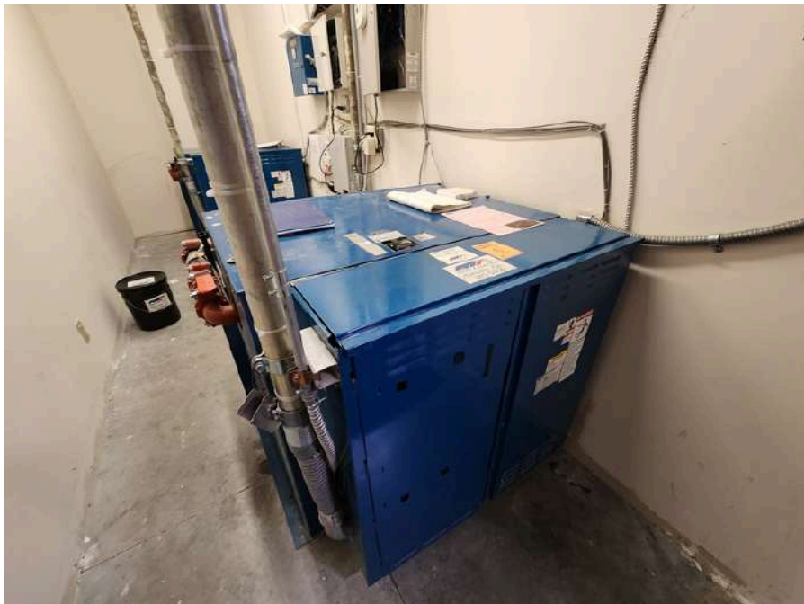
12. Elevator equipment at 8470
