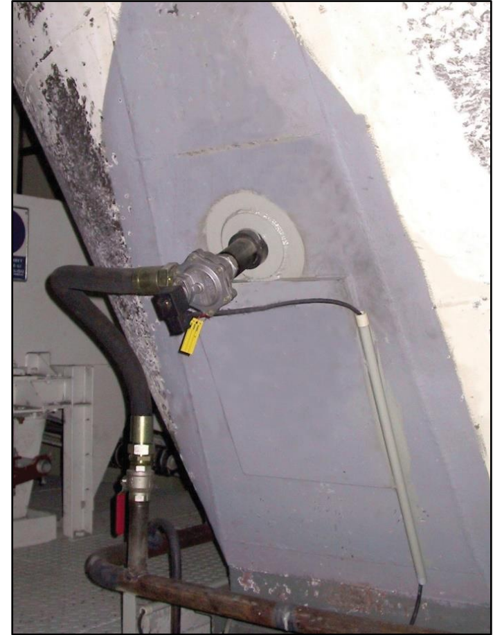
Model VA-51 on gypsum hopper
