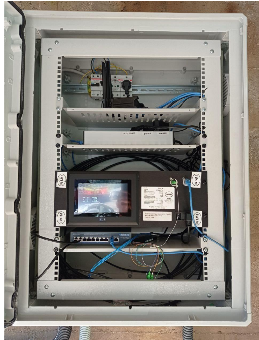
Figure 11: Datalogger dentro del housing
