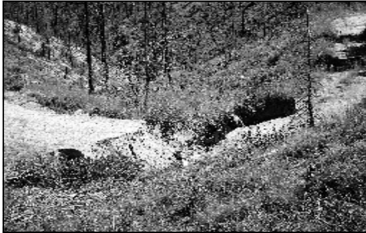
A washed-out road in the Boise National Forest, Idaho. RSP Photo
