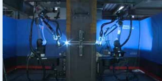
Coworking with autonomous robots. The robo-welder is among the three autonomous robots, equipped to operate on their own and work alongside people in Shimizu's Smart Sites (photo provided by Shimizu Corporation).
