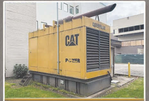
SPECIALTY AUCTION: CAT 3508 750KW DIESEL GENERATOR MAY 6, 2026
