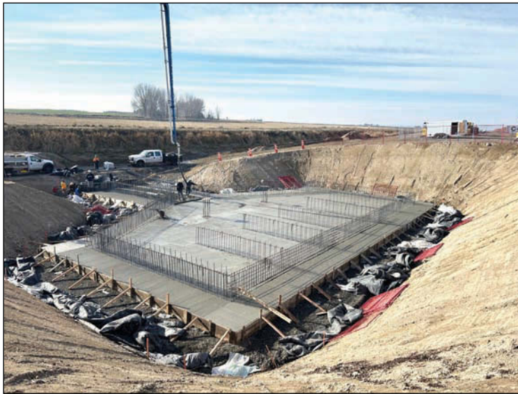
Construction on the Columbia Basin Project. (Courtesy East Columbia Basin Irrigation District)
