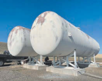
(2) 12,000 GAL NH3 TANKS, Blackmer Pump.....$14,500
